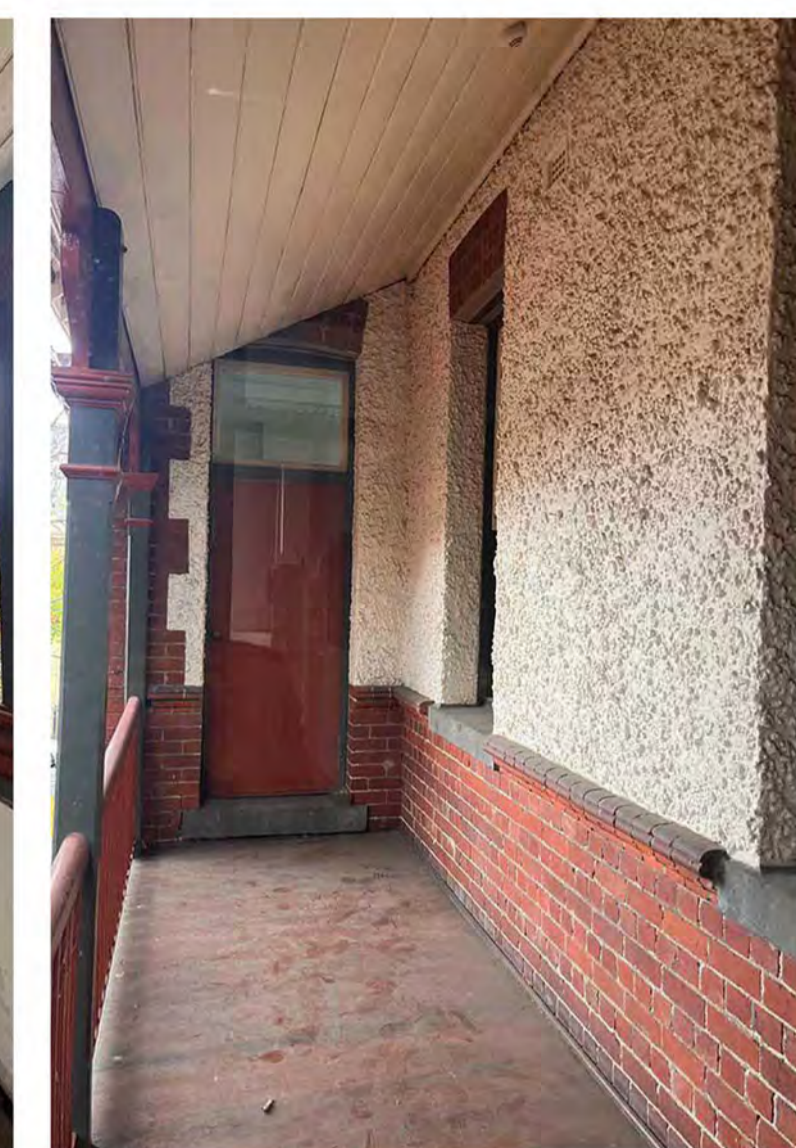
SITE PHOTO #6 • LEVEL 01 NORTH VERANDAH NON-COMPLIANT DUE TO FLOOR SLOPE AND LOW BALUSTRADE. ALLOWS FALLING DANGER.
