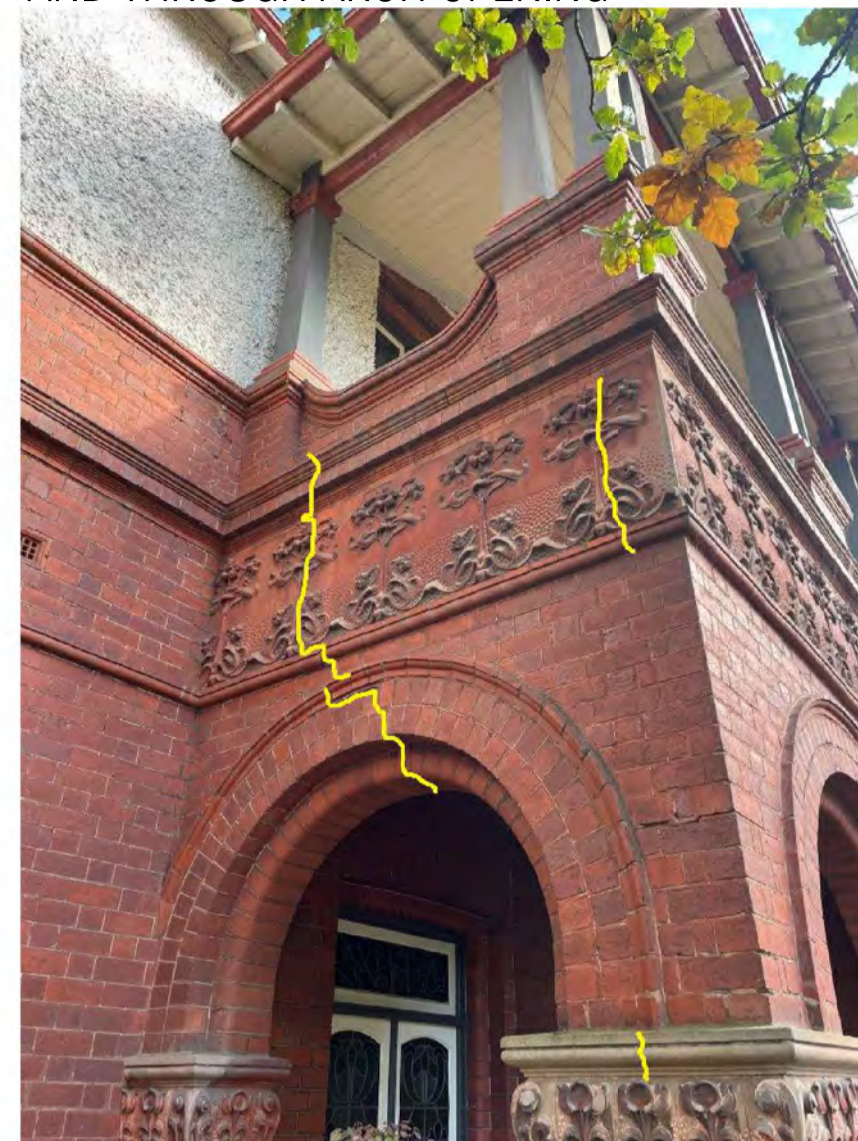
STRUCTURAL CRACK TO WALL. AND THROUGH ARCH OPENING
