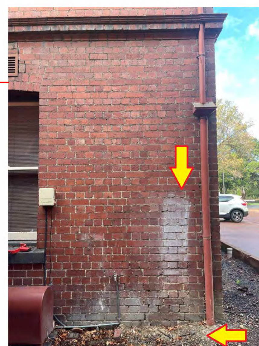
RISING DAMP NOT ENOUGH SUB-FLOOR VENTILATION
