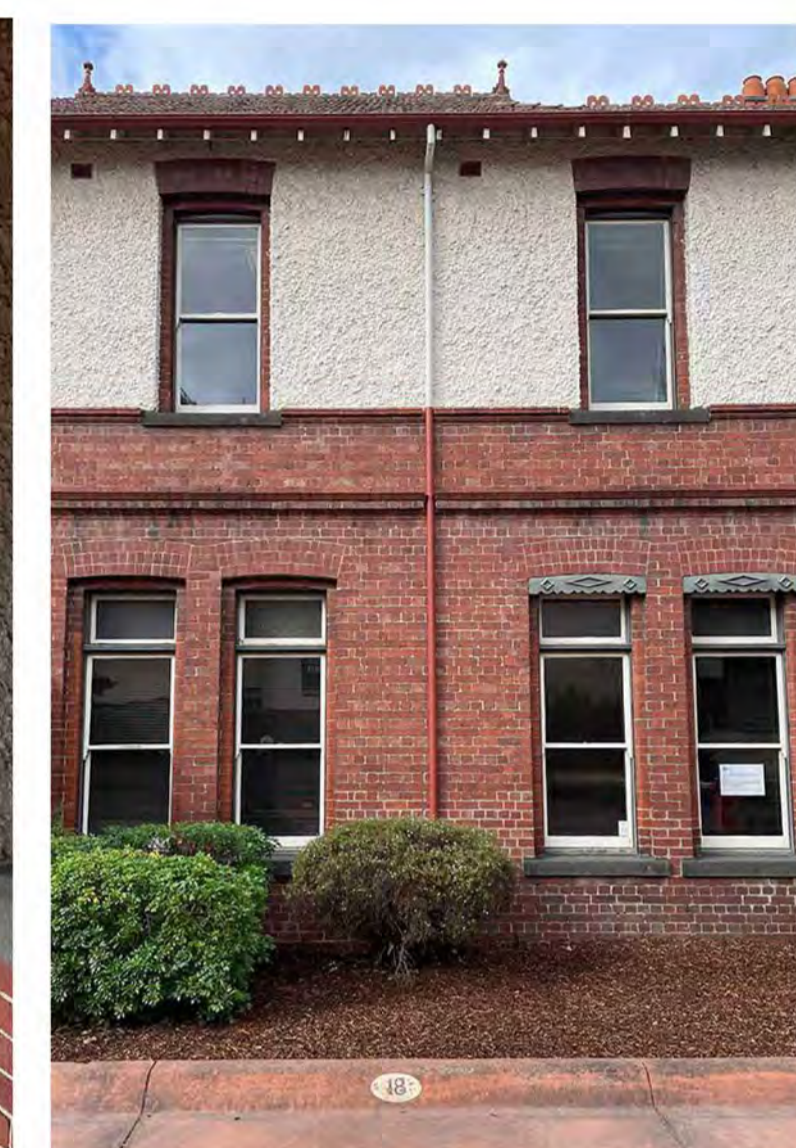
SITE PHOTO #7 • ENERGY EFFICIENCY TO EXISTING SINGLE GLAZED WINDOWS NON-COMPLIANT.
