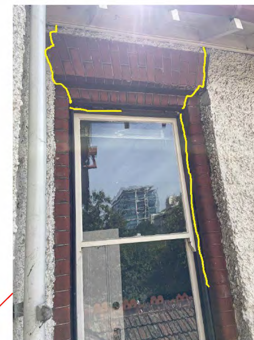
BRICK LINTEL SEPARATING
