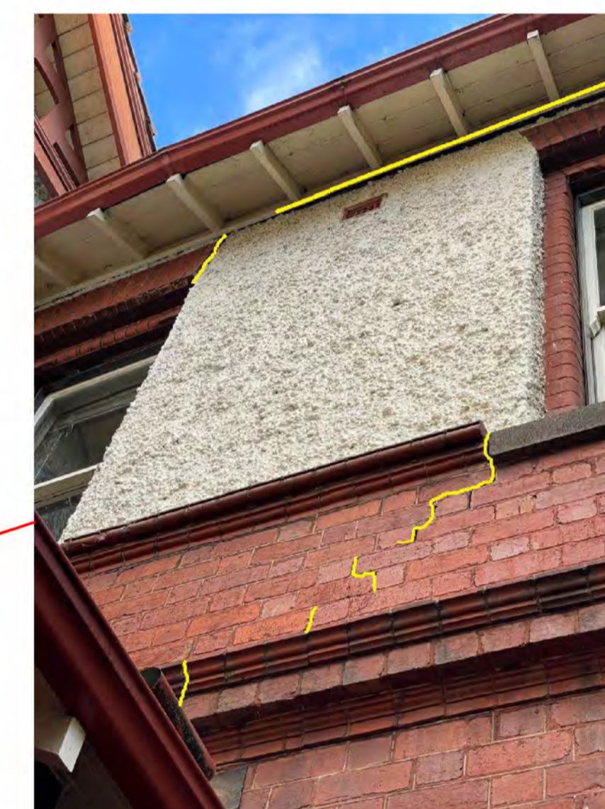
LARGE GAP BETWEEN SOFFIT AND WALL CLADDING
