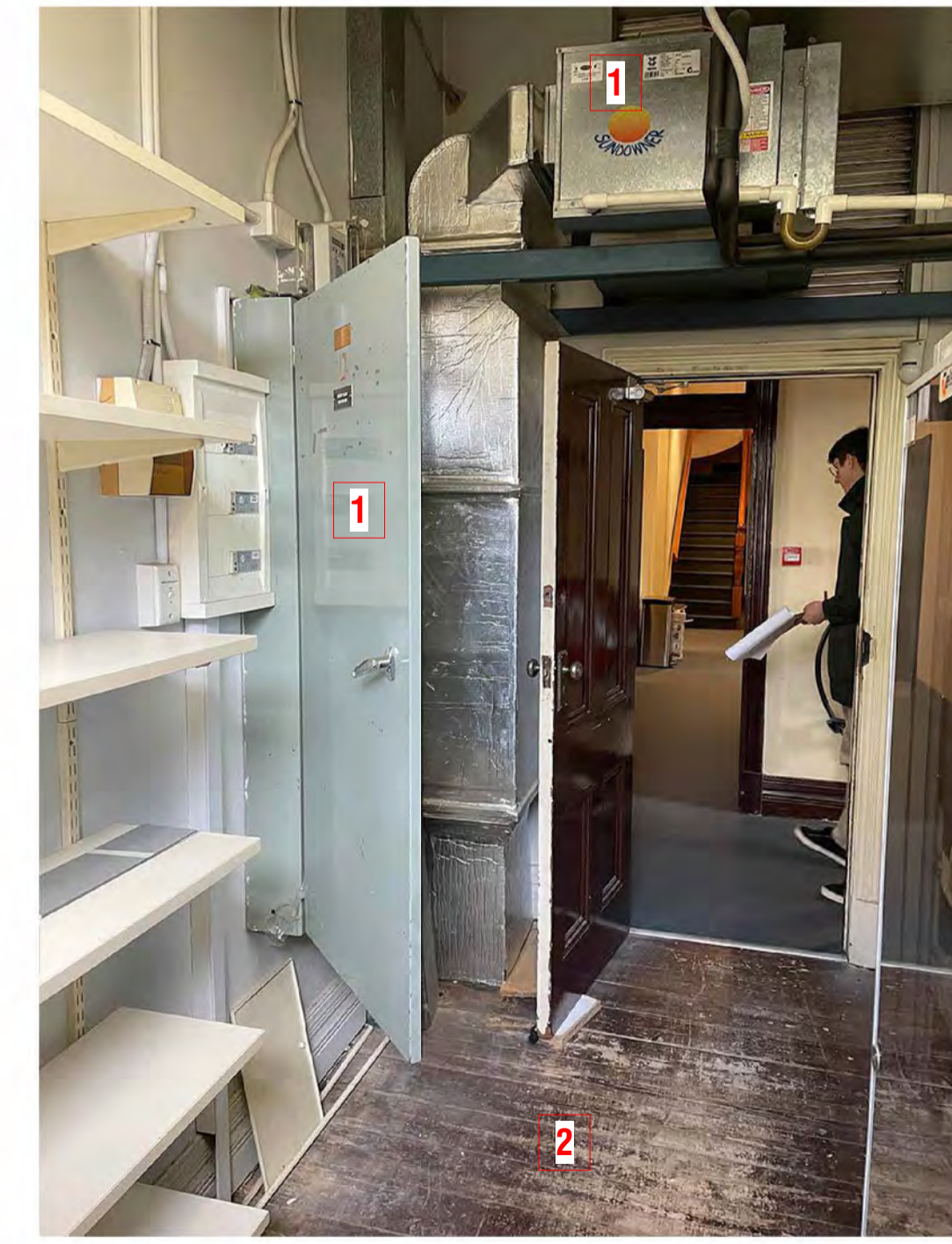
PHOTO - VIEW INTO AC DUCT ROOM
