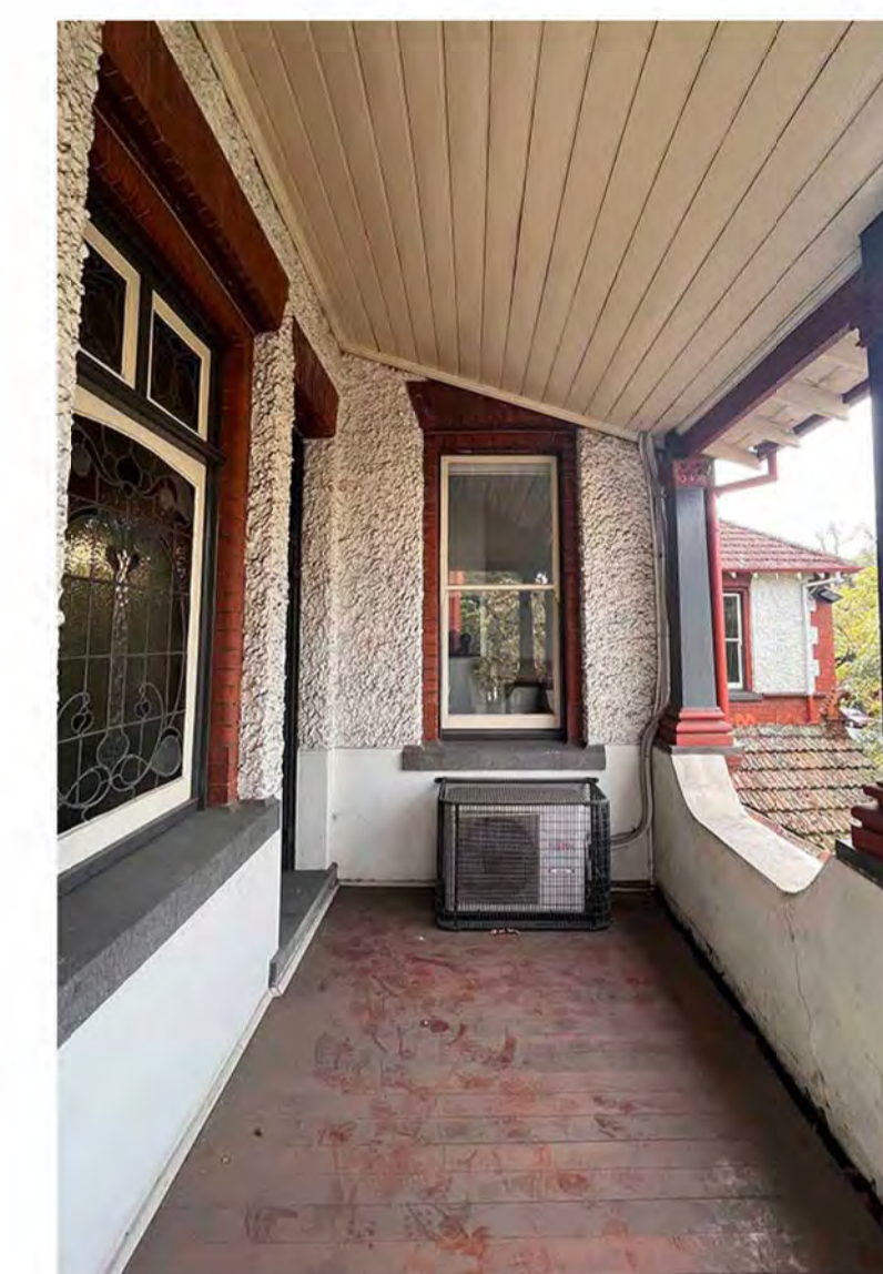
SITE PHOTO #5 • LEVEL 01 FRONT VERANDAH DOES NOT COMPLY DUE TO FLOOR SLOPE AND RAILING HEIGHT. DOES NOT HAVE COMPLIANT WATERPROOFING
