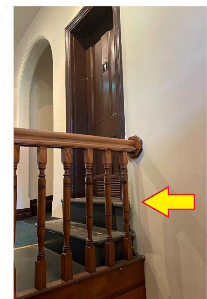
SITE PHOTO #1 • REMOVE STAIR & NON-ORIGINAL WC ON LANDING TO OPEN UP WINDOWS TO HALLWAY. • EXTG. STAIR BALUSTRADE NON-COMPLIANT. HANDRAIL TOO LOW. • REMOVE NON-ORIGINAL FLOORING.
