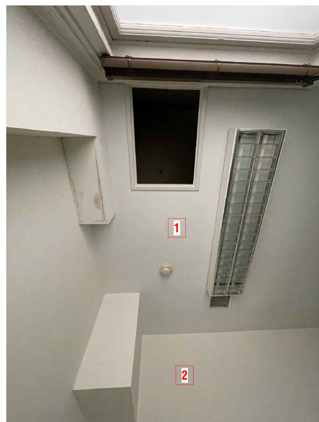
PHOTO - CURRENT URINAL CEILING
