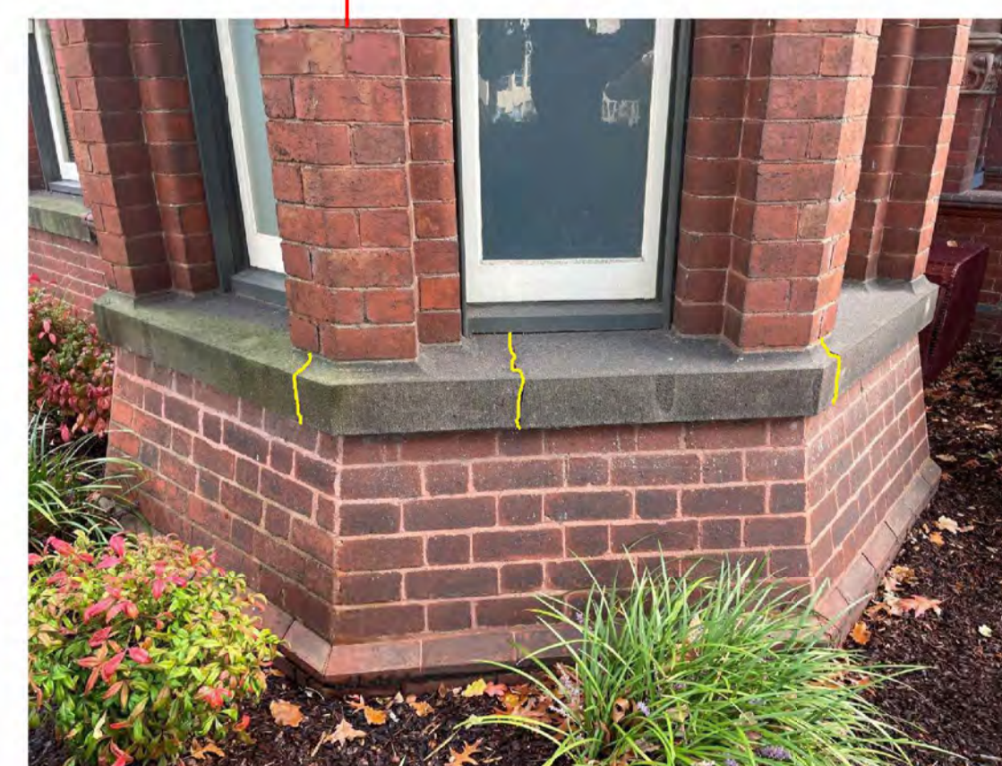
CRACKED SILL AROUND BAY WINDOW
