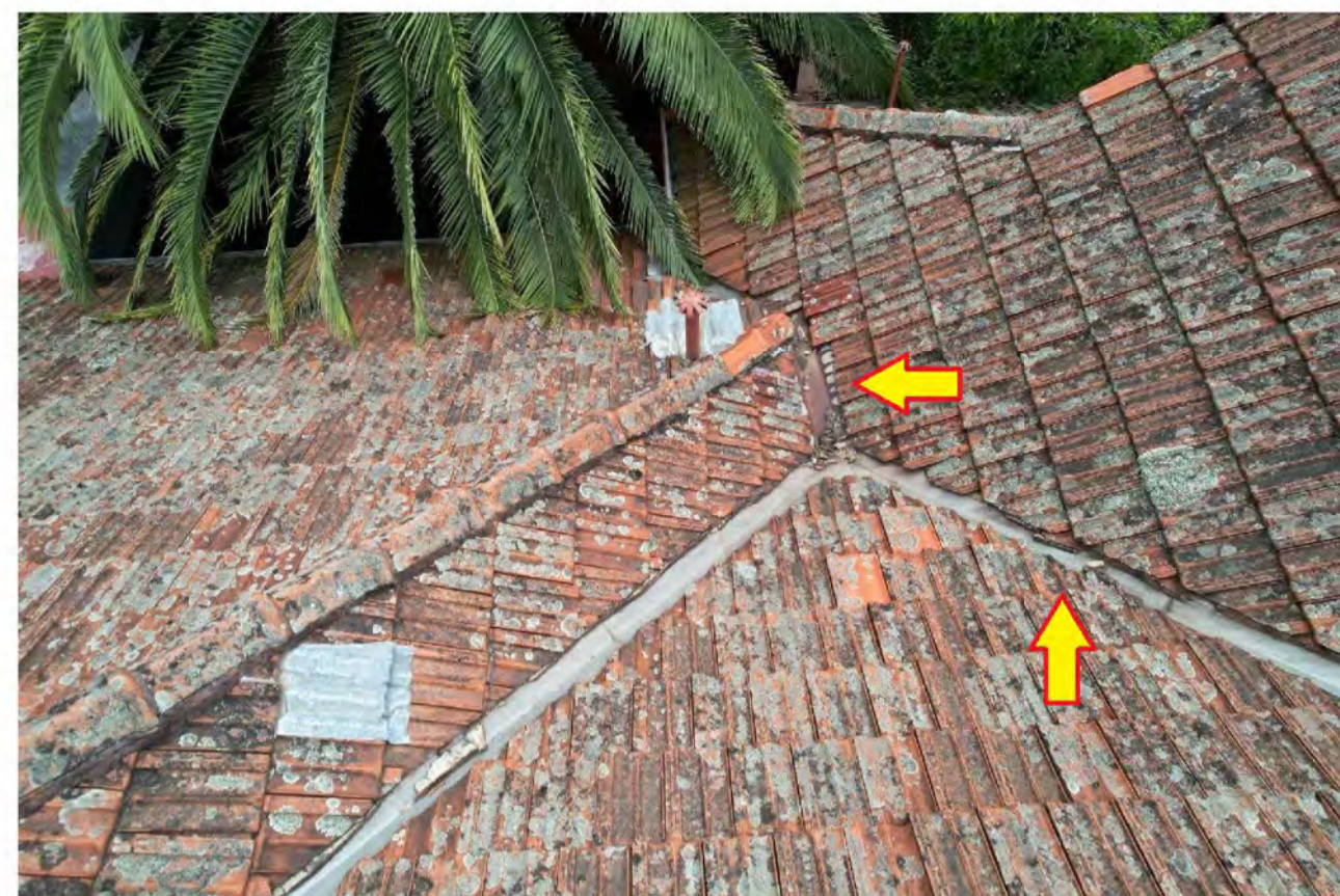
NOT ENOUGH CLEARANCE FOR VALLEY GUTTERS DEBRIS IN ROOF GUTTER BLOCKING DRAINAGE
