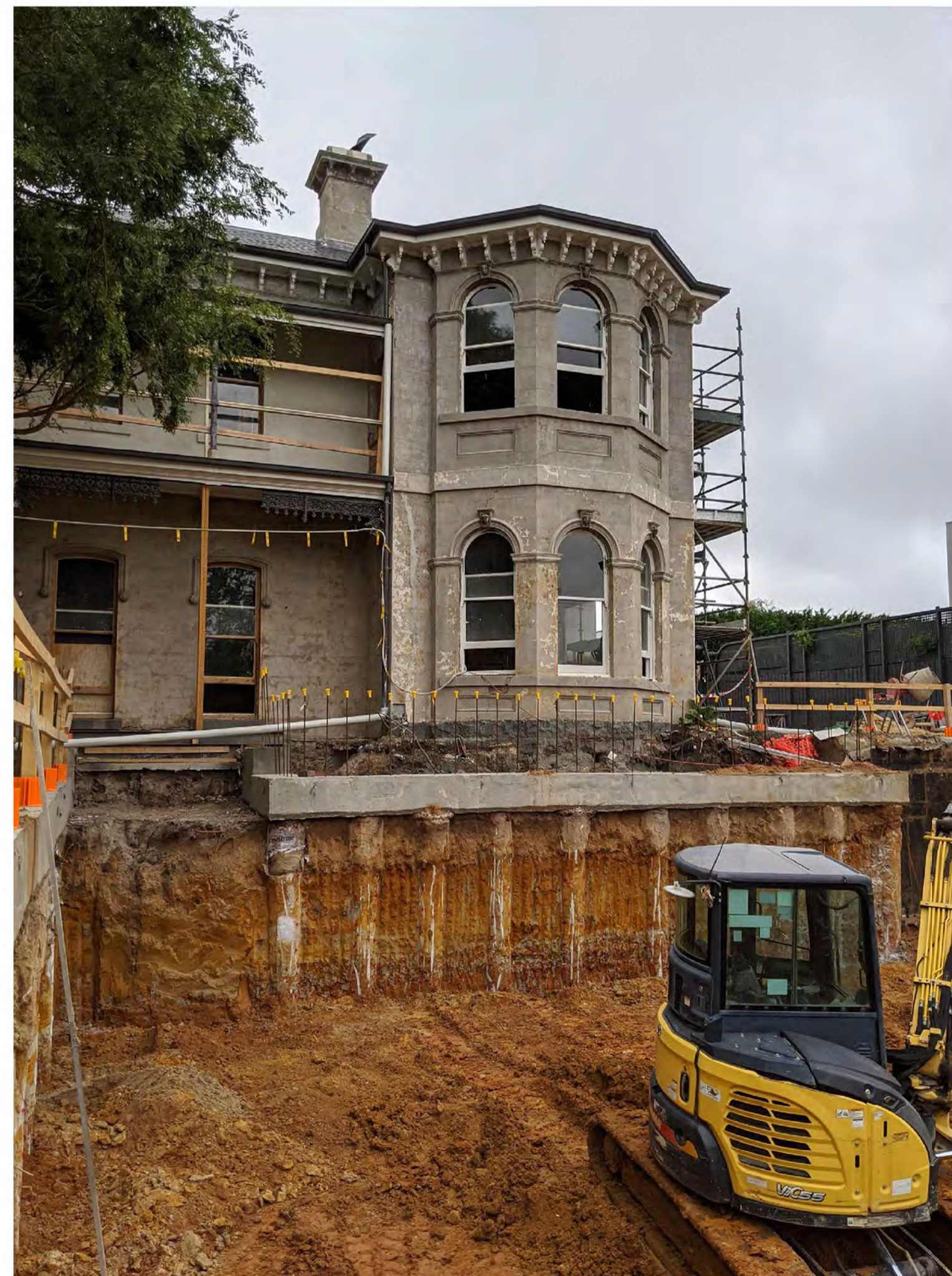
REFERENCE PHOTO - BASEMENT RETENTION WORKS OUTSIDE OF EXISTING HERITAGE HOUSE. CAPPING BEAM AND BORED PIERS INSTALLED
