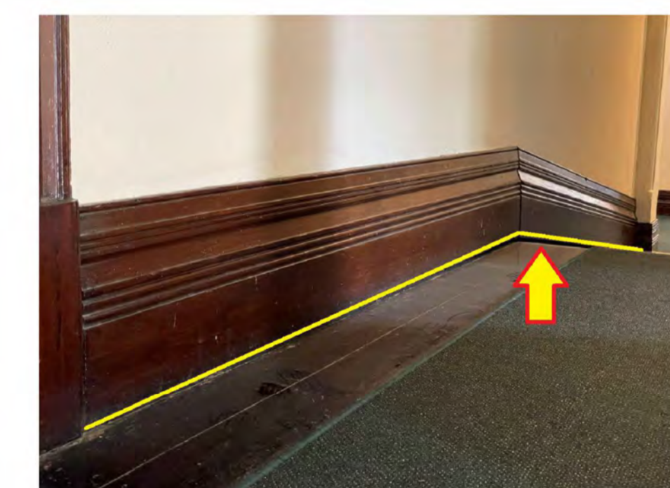
SITE PHOTO #4 - FIRST FLOOR RAMP • EXISTING RAMP GRADIENT TOO STEEP. TRIP HAZARD • LARGE GAPS BETWEEN SKIRTING TO FLOOR BOARDS
