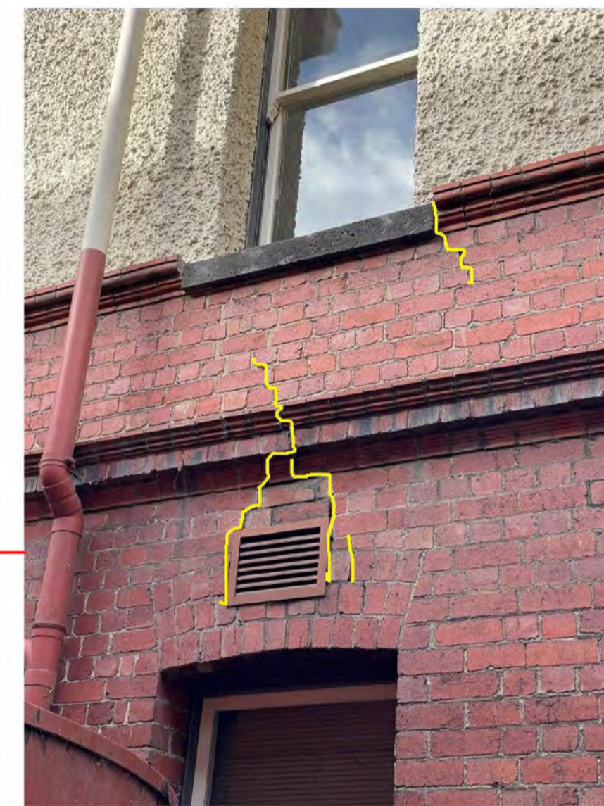
CRACKING IN MASONRY WALL
