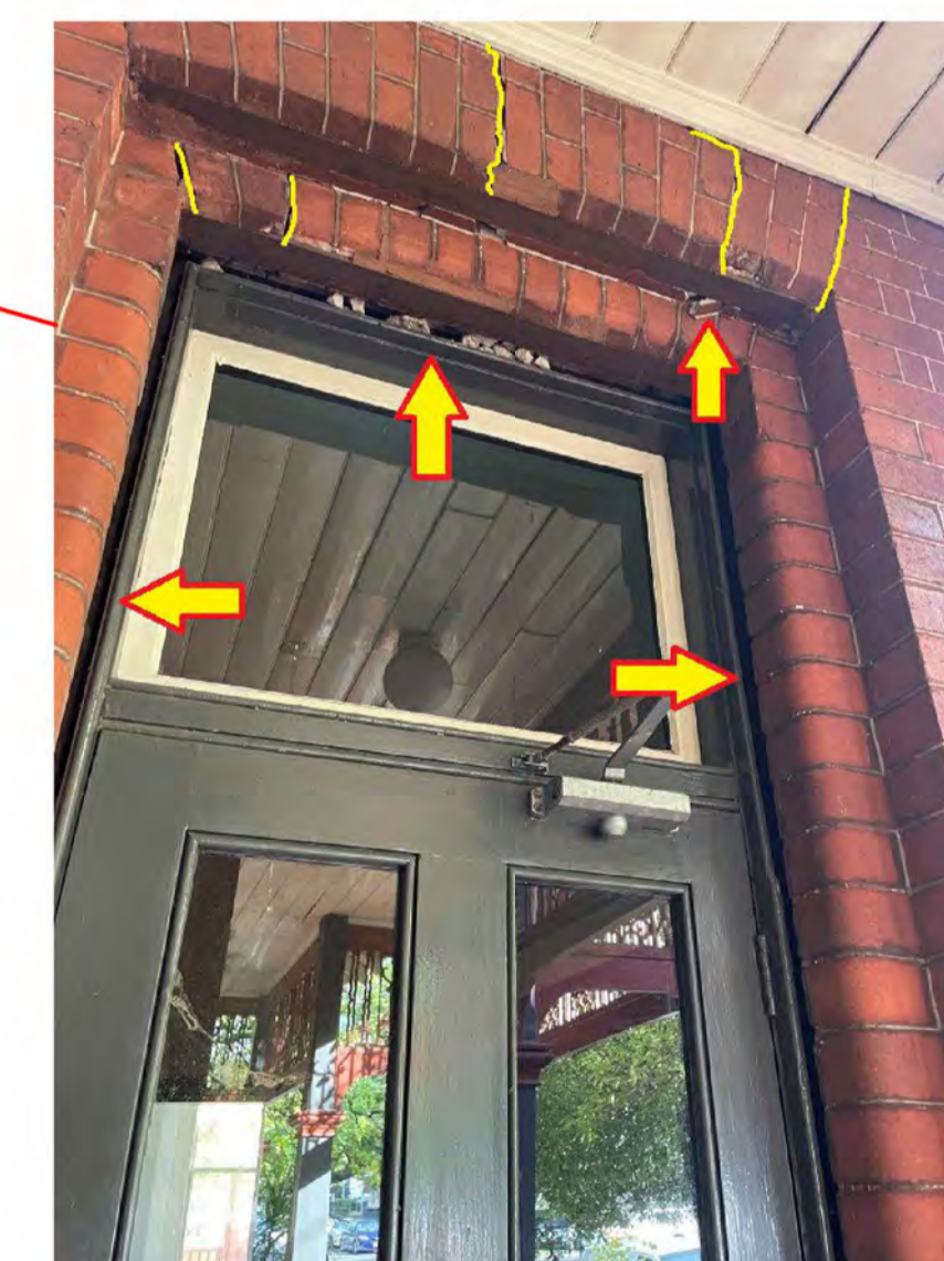
BRICK LINTEL CRACKING. DOOR LEANING / PEELING AWAY FROM OPENING
