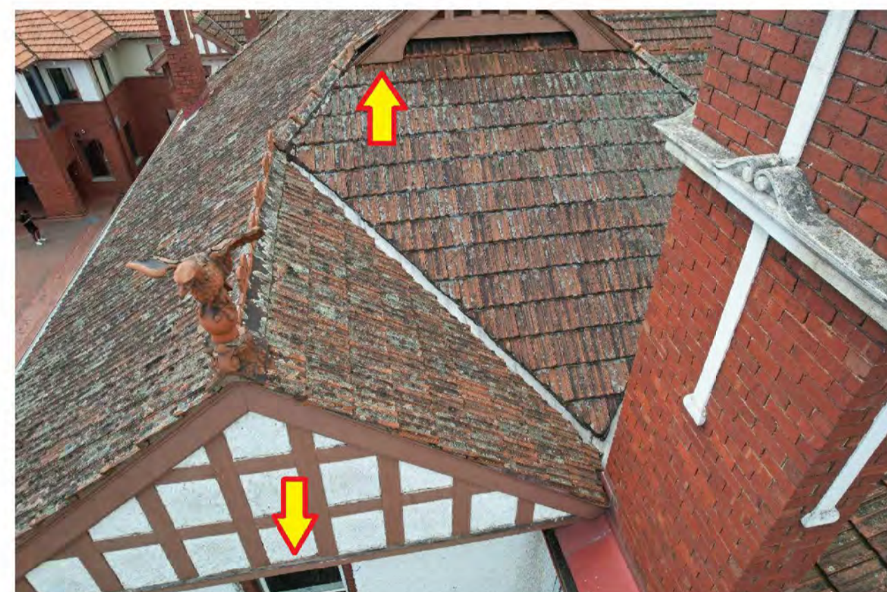
TIMBER STRAPPING SHOWING SIGNS OF ROT. REPAIR REQUIRED
