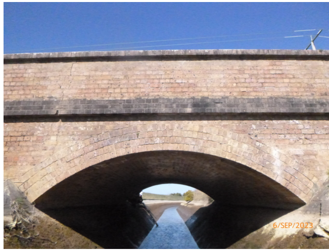
DEFECT 24: FULL VERTICAL CRACK ON THE NORTHERN SPANDREL WALL TOWARDS EAST ABUTMENT
