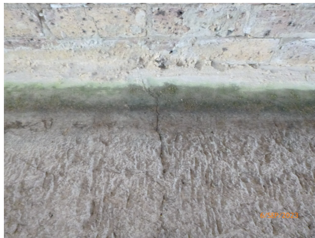
DEFECT 27: VERTICAL CRACK NOTED ON EAST FACE OF AQUEDUCT AT MIDSPAN
