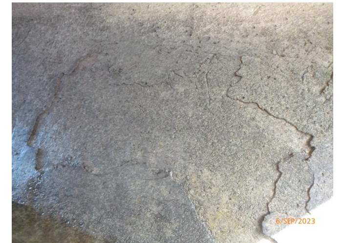
DEFECT 26: SPALLING OF CONCRETE 1300MM X 500MM ON WEST FACE WATERWAY INVERT PROTECTION
