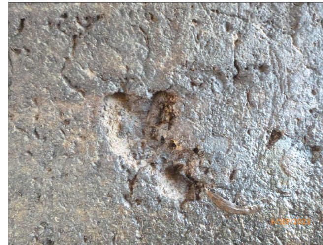
DEFECT 26: SPALLING OF CONCRETE ON EAST FACE WATERWAY INVERT PROTECTION
