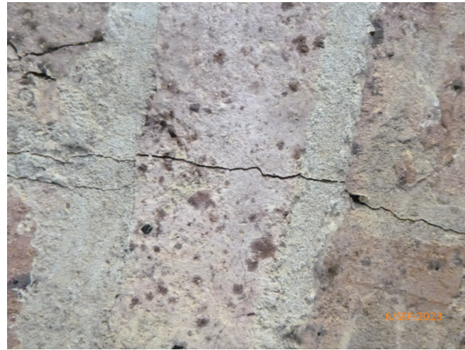
DEFECT 21: LONGITUDINAL CRACK AT MIDSPAN OF THE BRIDGE ACROSS ENTIRE LENGTH
