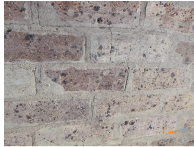
DEFECT 22: LONGITUDINAL CRACK FROM SOUTH ELEVATION ON WESTERN FACE OF ARCH
