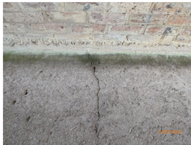
DEFECT 27: VERTICAL CRACK NOTED ON WEST FACE OF AQUEDUCT AT MIDSPAN
