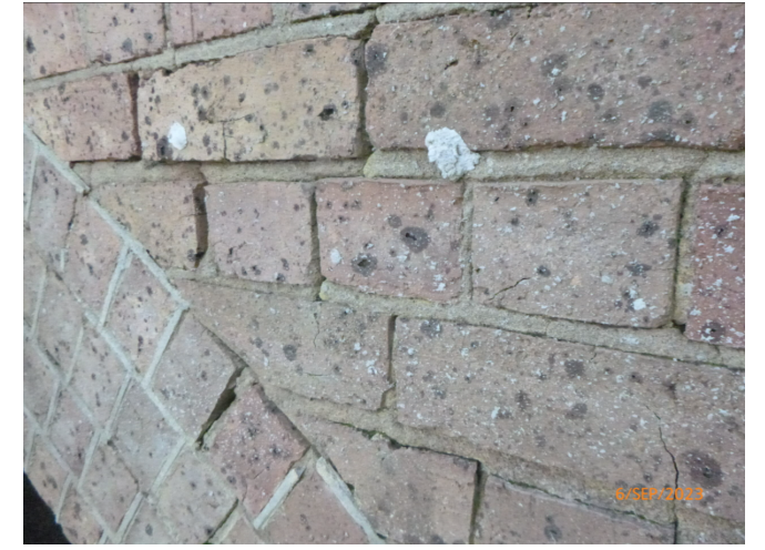
DEFECT 23: MORTAR LOSS BELOW WEST PARAPET ON SOUTH FACE OF RCH BRIDGE
