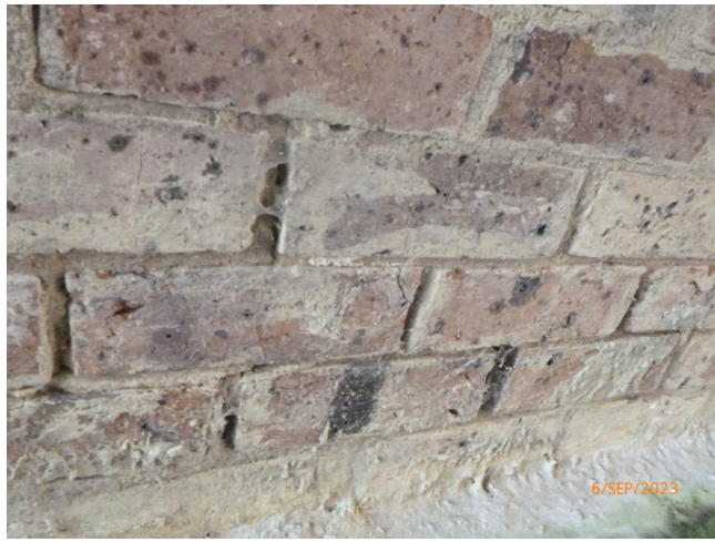
DEFECT 20: MORTAR LOSS ON THREE LAYERS OF BRICKS ABOVE WEST WATERWAY INVERT PROTECTION
