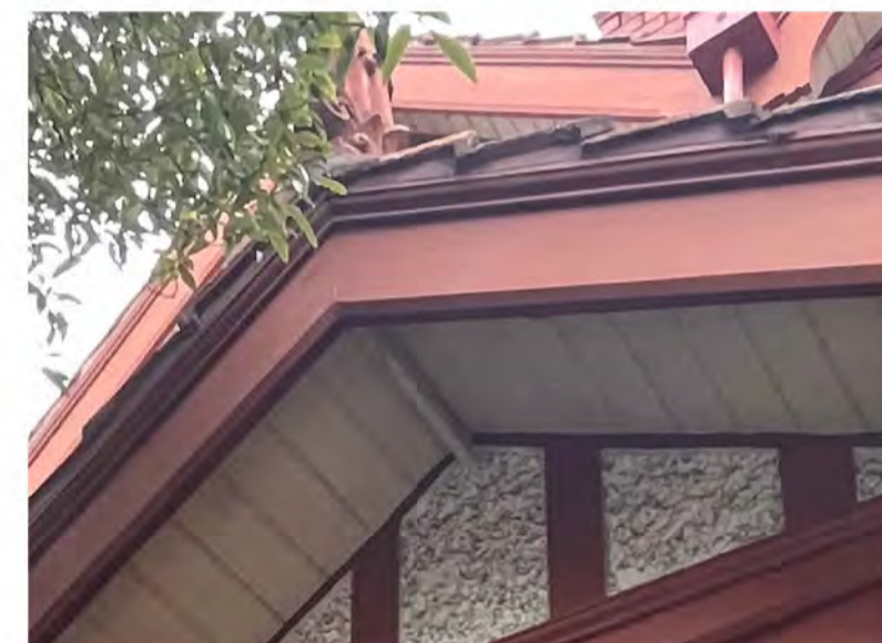
GABLE END FASCIA BOARD CHECK FOR DECAY, TREAT ROT WHERE REQUIRED. PATCH AND PAINT COLOUR TO MATCH EXISTING
