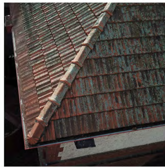
EXISTING ROOF RETAINED CHECK TERRACOTTA TILES FOR CRACKS, SLIPPAGE, BROKEN TILES, AND MISSING FLASHING. MAKE GOOD ROOF TILES, CAPPING AND FLASHINGS. REPLACE TO MATCH EXISTING AS REQUIRED
