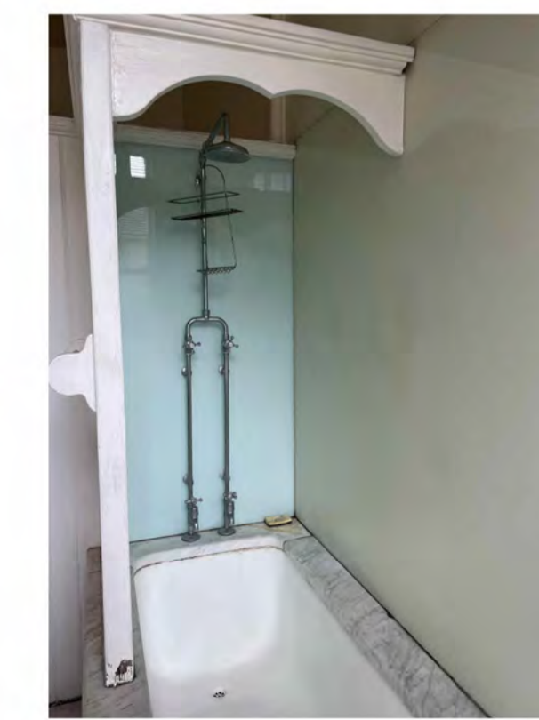
NON-ORIGINAL SHOWER SURROUND (GLASS SPLASHBACK) AND FITTINGS TO BE REMOVED
