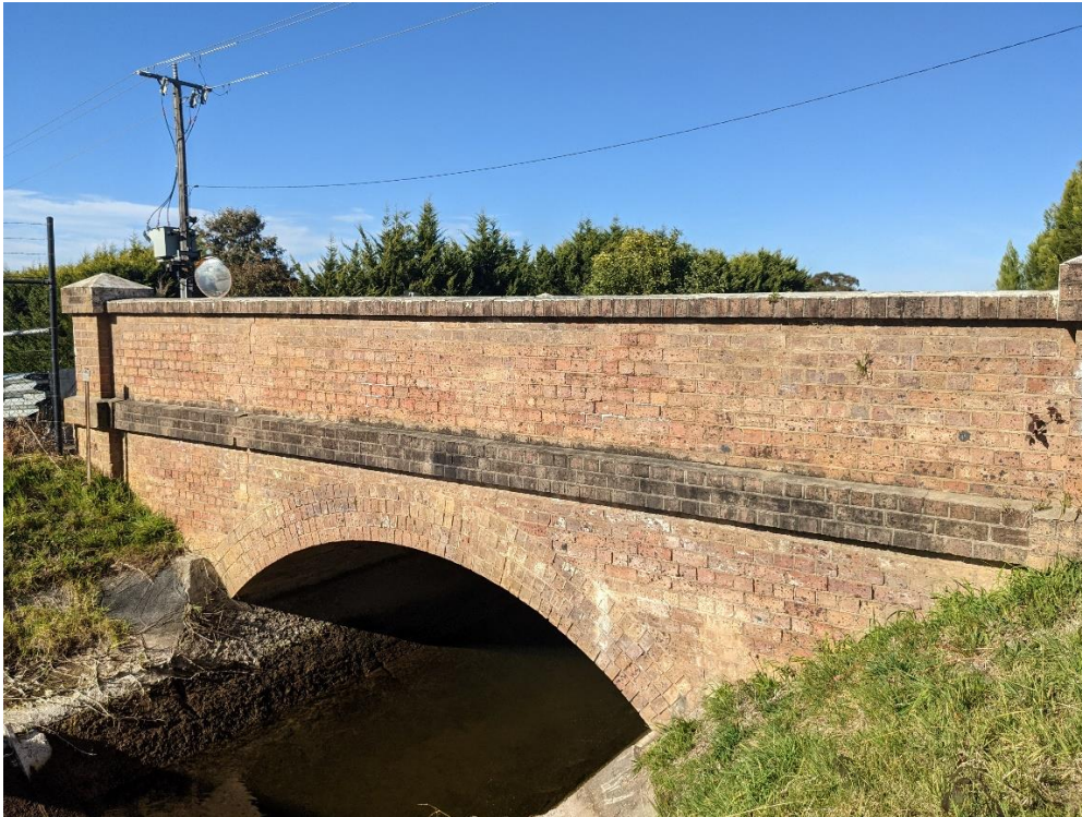
Figure 4.2 Northern side of the bridge, showing its simple vaulted arch form. (Source: GML August 2023)
