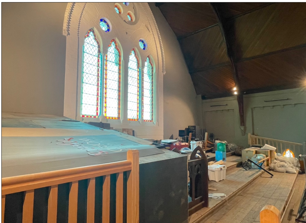
Figure 7 The gallery. It is proposed that the Fuller organ be installed in two sections either side of the stained glass window.
