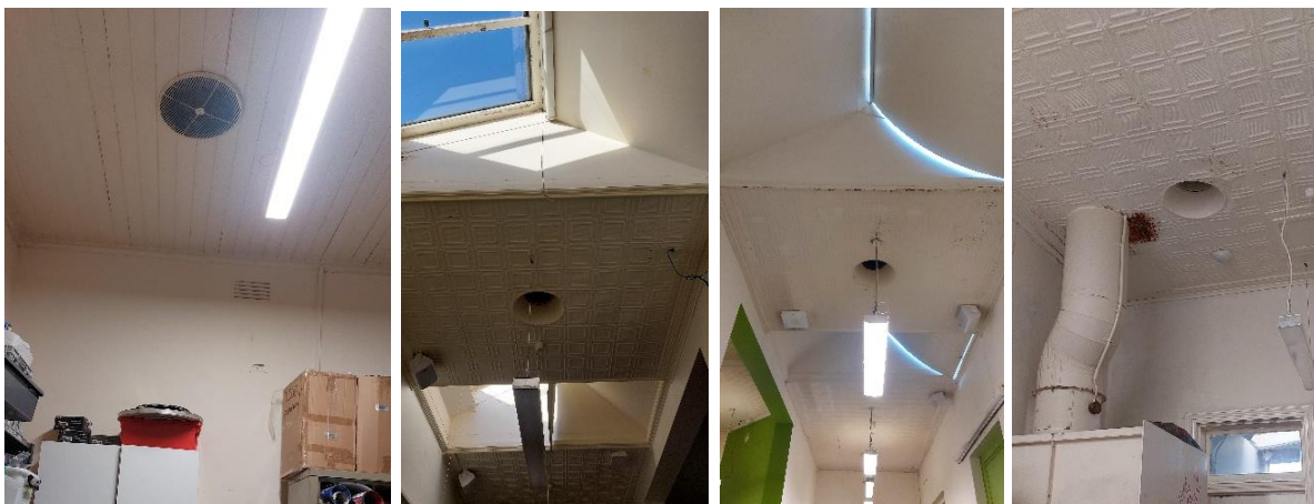
Figure 6: Ceiling mounted exhaust fans, and skylights with manually operable shades.
