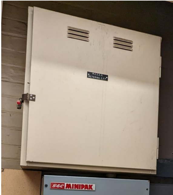
Figure 9: CT Metering Enclosure
