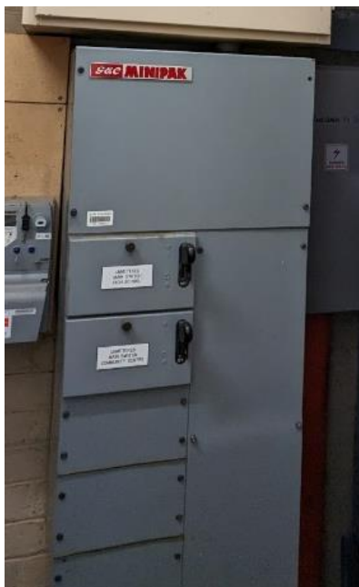
Figure 8: Main Switch Board
