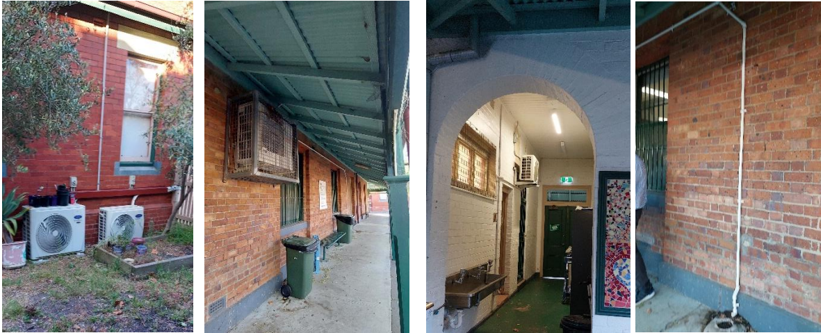
Figure 4: From left, Outdoor installation for the existing split ACs, and condensate drainpipe termination to a floor gully.
