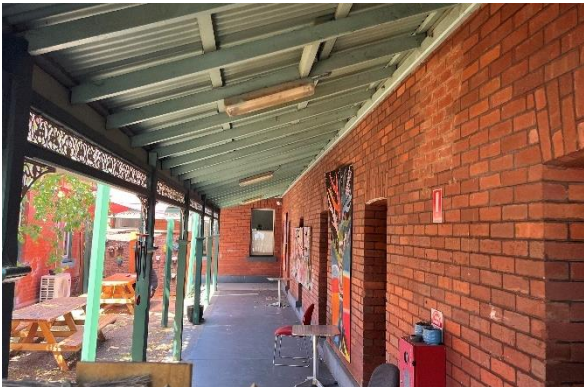
Figure 33. Internal verandah of the southern wing to the C shaped building, looking east.
