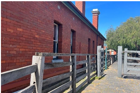
Figure 30. Partial view of the southwestern elevation, looking southeast, with the existing ground placed HVAC unit is obscured by fencing.
