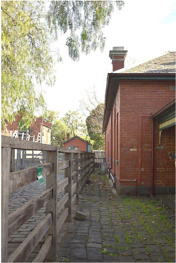
Figure 28. Looking northwest along the southwestern elevation of B1(2). The image shows the existing ground placed condenser.
