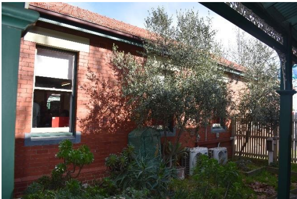
Figure 37. Partial oblique view of the northern elevation to B1(2) central building, including existing HVAC services located on the ground and behind the fence.
