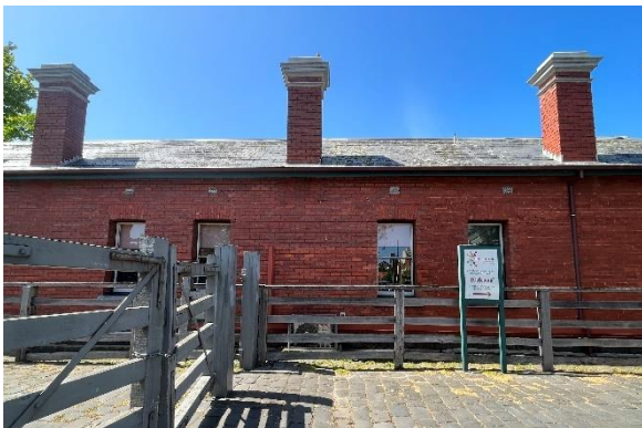
Figure 29. Partial view of the southwestern elevation, with the existing ground placed HVAC obscured by fencing.
