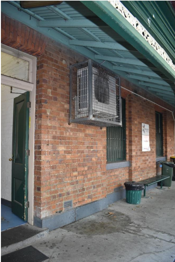
Figure 22. The existing mounted HVAC unit to the southwestern elevation.
