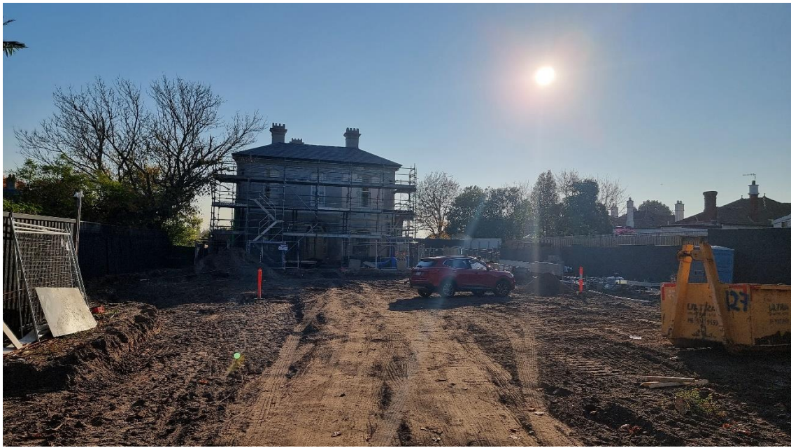
Figure 7: Front setback of the house, note scaffolding remains in place and landscaping works are ongoing. Source: Trethowan Architecture, 2024.
