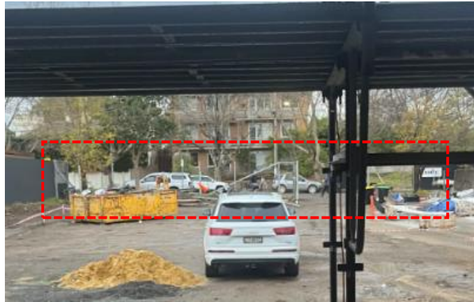
Figure 9: View from the verandah, note temporary construction hoarding has been removed (indicated in red) whilst endorsed fence design is under construction. Source: Courtesy of client, 2024.
