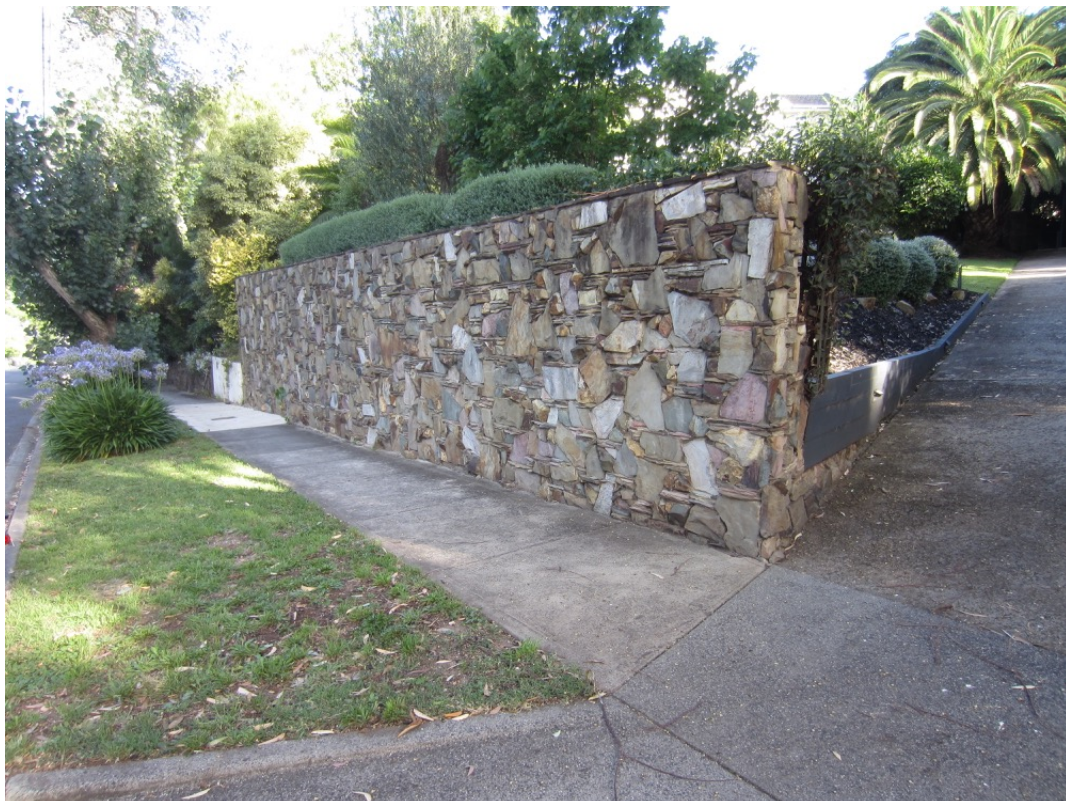
Figure 3 View of the stone retaining wall/fence along Carlsberg Road to the east of the driveway.
