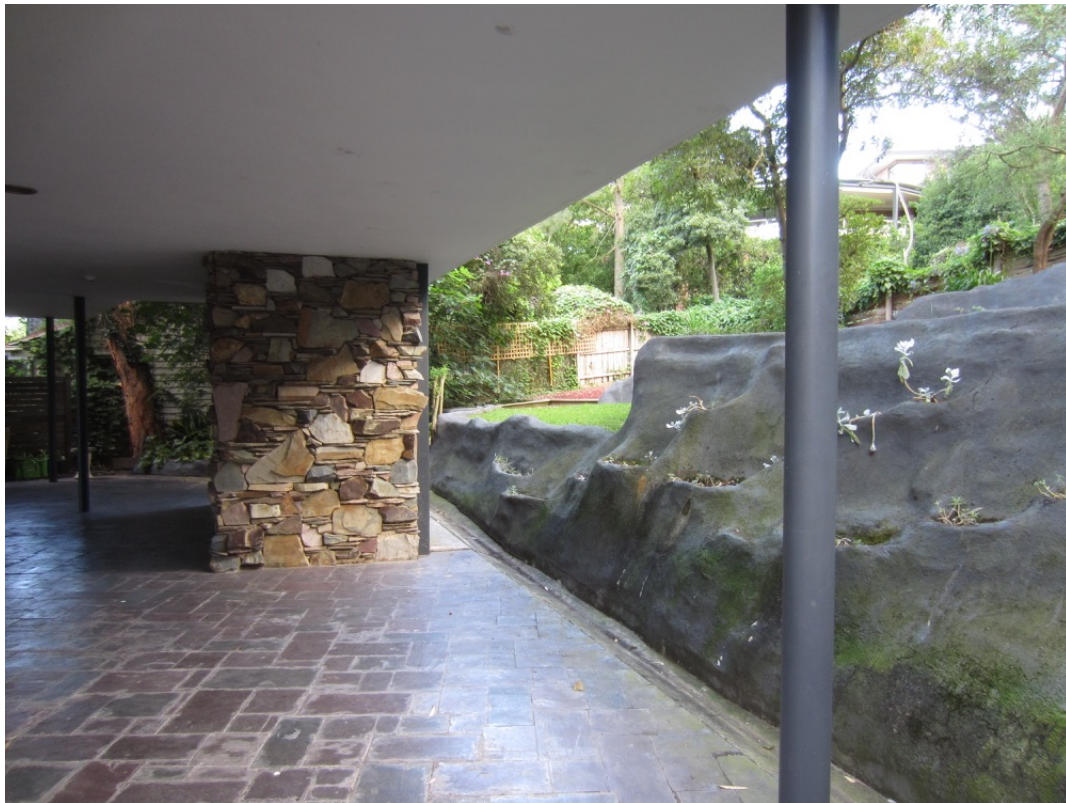
Figure 12 Rear of the undercroft showing the free form cement render on brick retaining wall with planter pockets. The retaining wall was added later to stabilise the cut slope.
