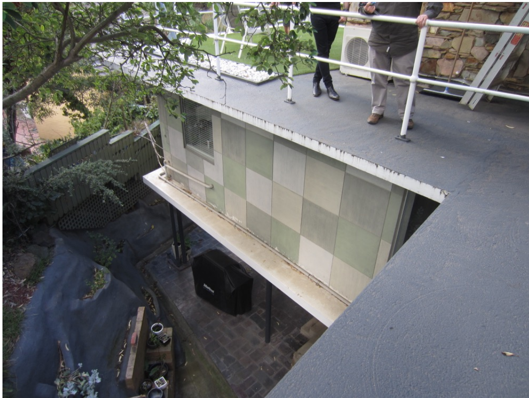
Figure 16 View from the second storey showing the south wall and garden retaining wall.
