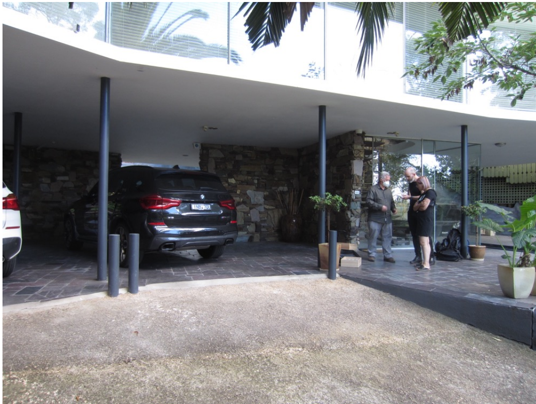
Figure 10 The undercroft entrance to the house showing the slender steel piloti and stone clad walls supporting the first floor concrete slab.
