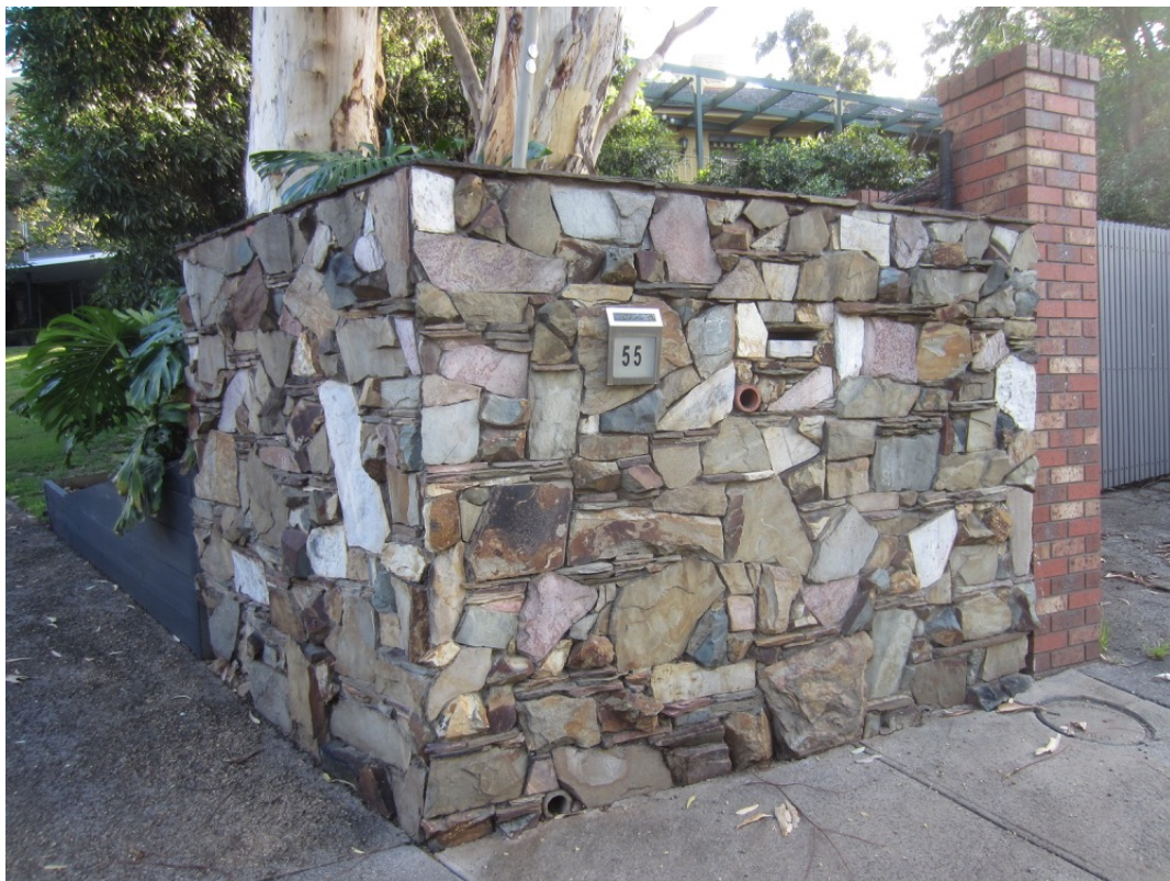
Figure 5 West part of the stone retaining wall/fence to the west of the driveway.
