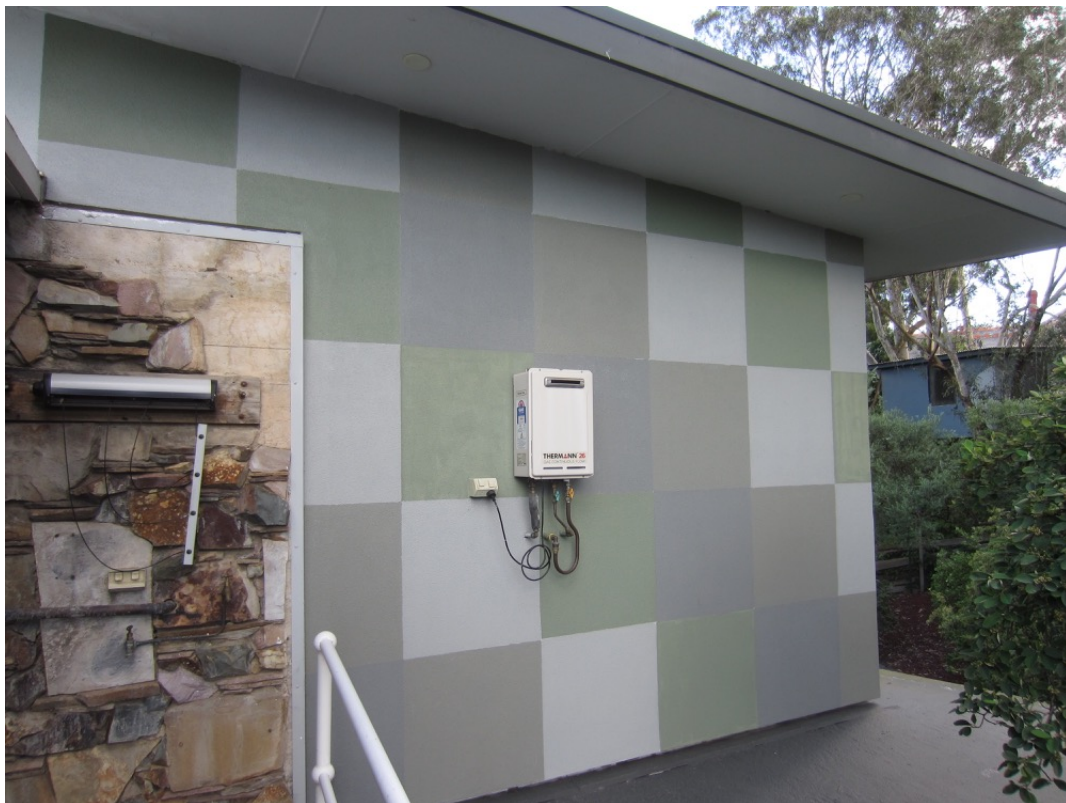
Figure 15 Part view of the west wall of the 2016 second storey addition with an interpretation of the original decoration on the rendered cement sheet cladding.
