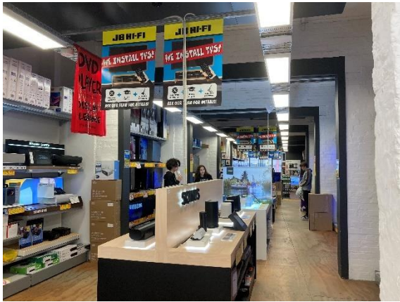
Figure 29: Cable trays and lighting to side bay
