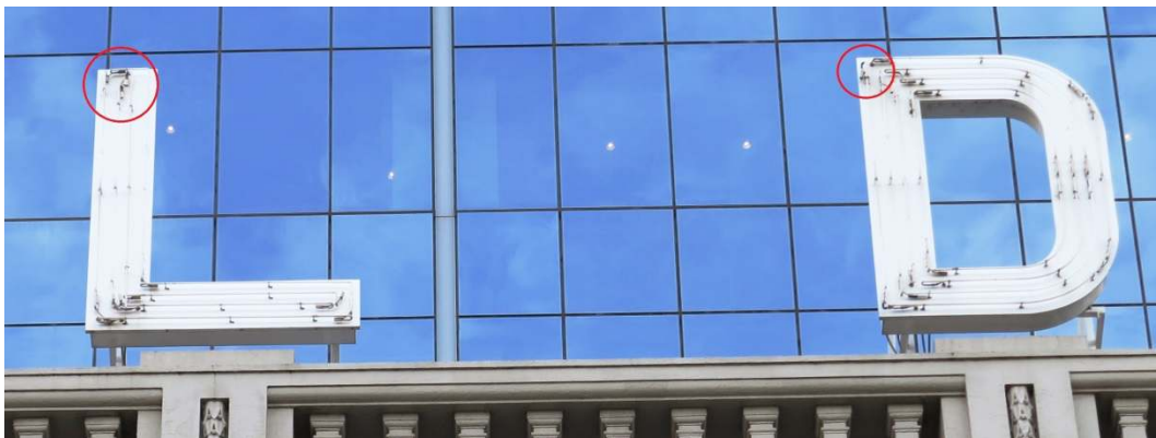
Letters L & D seen from Flinders Street Letters L + D with red circles indicating inlets in the letter boxes where wiring is presently taken through to internal transformers which convert the electric current into a higher voltage
