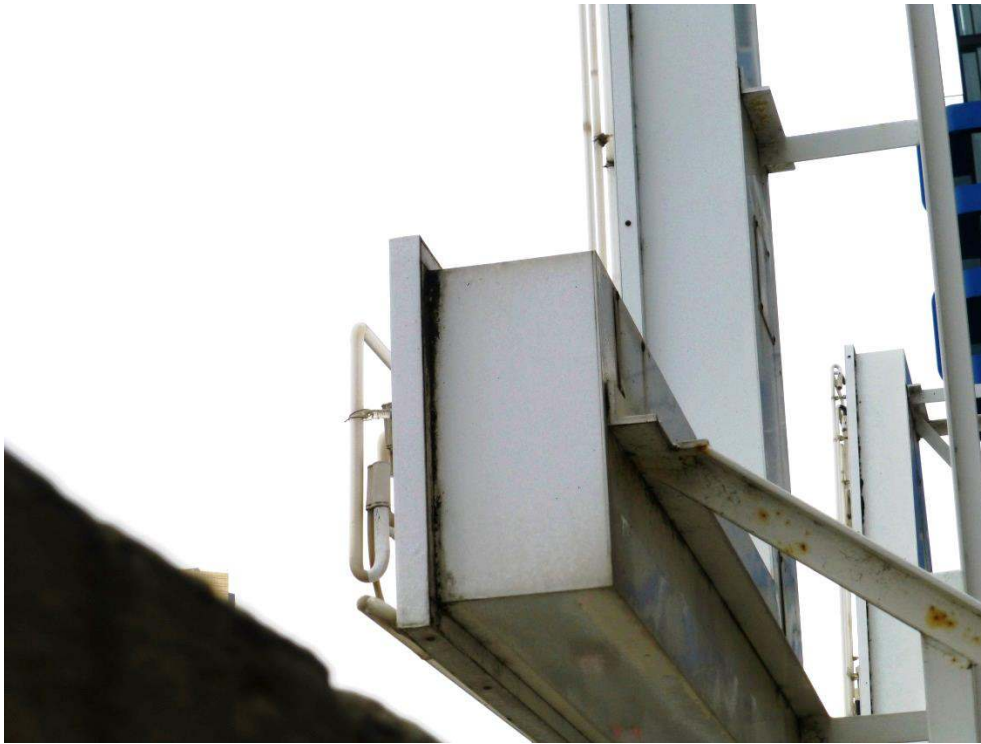
Letter edge: the new fascia will be clipped over the existing: it is proposed to remove the neon tubes
