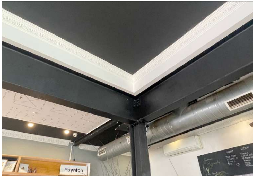
Figure 14 Modern steel beams supporting the ceiling to the former banking chamber. The decorative plaster cornice is presumed to be original.
