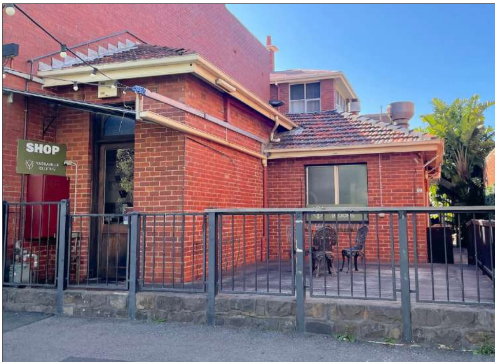
Figure 7 The post war additions viewed from Ballarat Street. The deck, balustrade and stone plinth are non-original.
