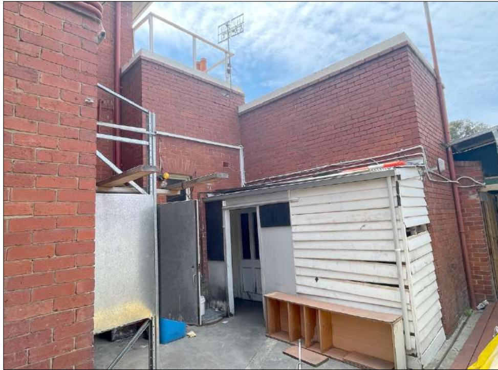
Figure 10 The eastern end of the south elevation showing timber lean-to abutting the rear service wing.
