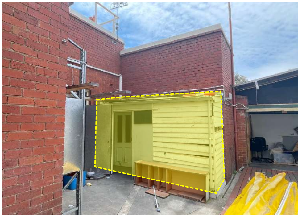
Figure 21 View of the rear wing showing the area where demolition works are proposed. This part of the building does not appear to date to the bank's original 1909 stage of completion.
