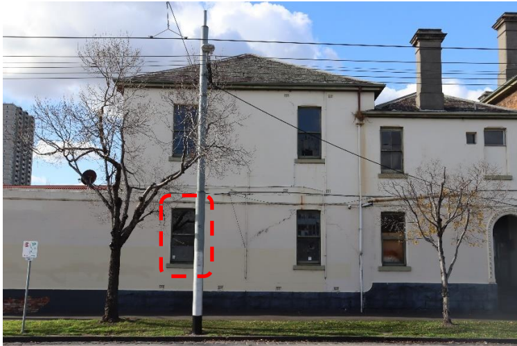
Montague Street elevation - rear service wing (1877). The highlighted window (dashed red) would become a blind niche.
