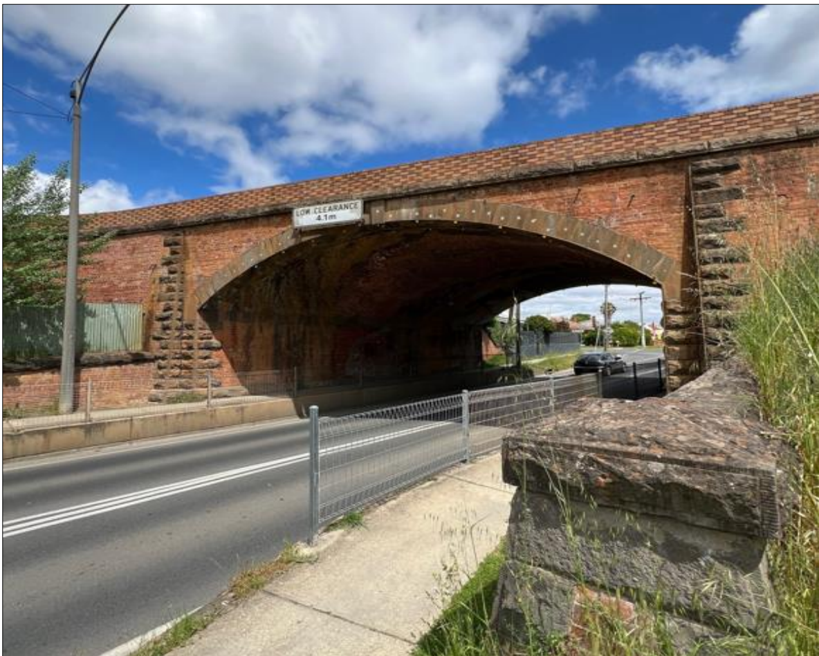
Fig.1. Facing east is original bridge with stone face arch voussoir and bluestone abutments (1862).
