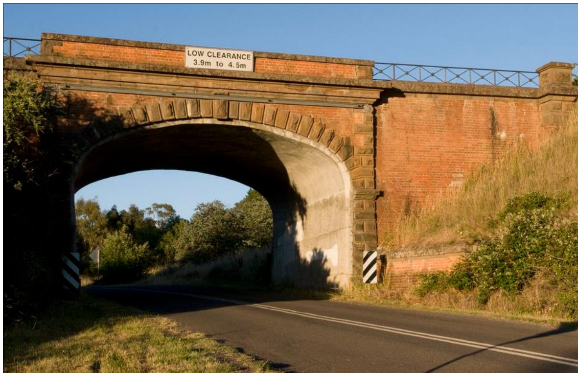
Fig.15. Fryers Rd Rail Bridge Chewton, (VHR H1780) with bridge soffit concrete lining installed in 1990. Note that this lining has not been colour tinted to match the overall structure.
