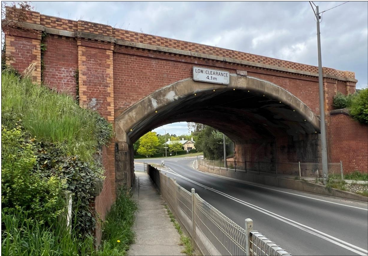
Fig.2 Facing west (1895 bridge extension) is the concrete lining 'voussoir' and barrel vault bridge addition with rectangular brick piers, wingwalls, and granite abutments.
