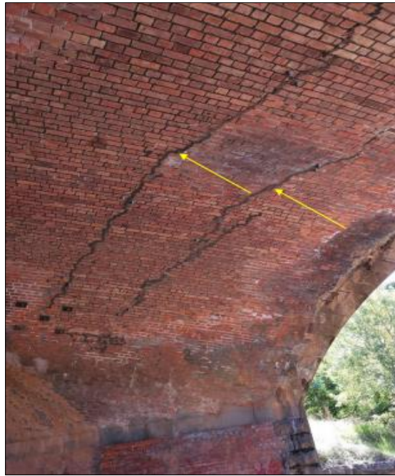
Fig.8. Longitudinal cracks along the arch soffit. 9
