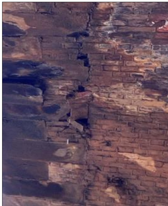
Fig.9. Deterioration of the bridge soffit at interface between concrete lining of the 1895 bridge and the red brick barrel vault of the original 1862 bridge. 10
