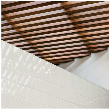
ROOF / SOFFIT LINING 1. SOFFIT BATTENS LIGHT TONES TIMBER SPOTTED GUM OR SIMILAR 2. ROOF SHEETING DANPAL ROOF SHEETING SYSTEM (T.B.C)
