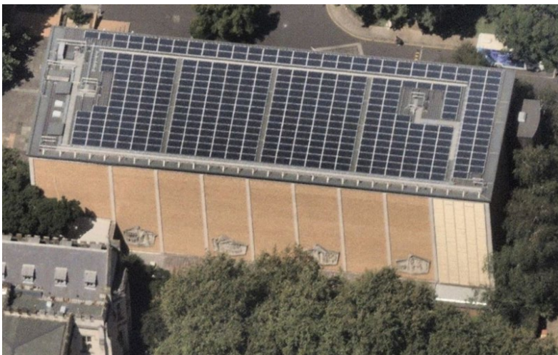
◀ Wilson Hall, aerial/panoramic view from west showing roof-mounted solar collectors. (Source: Nearmap. Image dated 3 February 2024)
