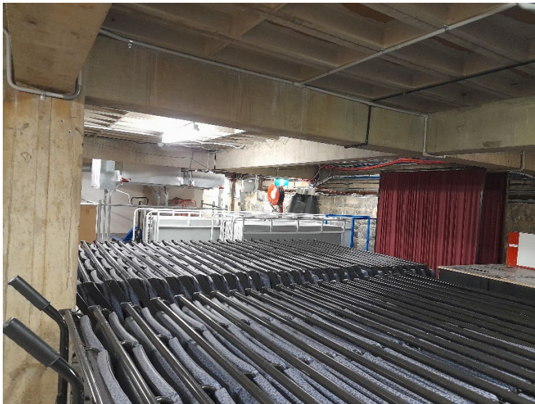
◀ Wilson Hall, basement. Stored seating. Note the limited headheight below the downstand beams.
