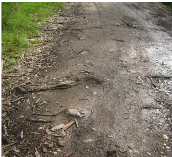
Figure 3. Large roots located under roadway
