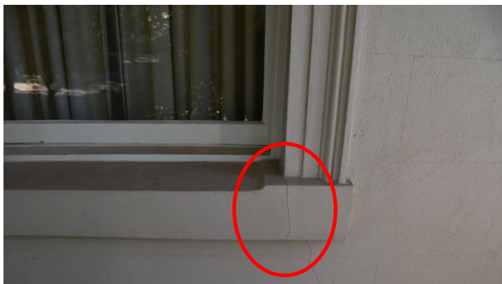
Figure 12 Hairline crack reportedly caused by the Ficus macrocarpa.
