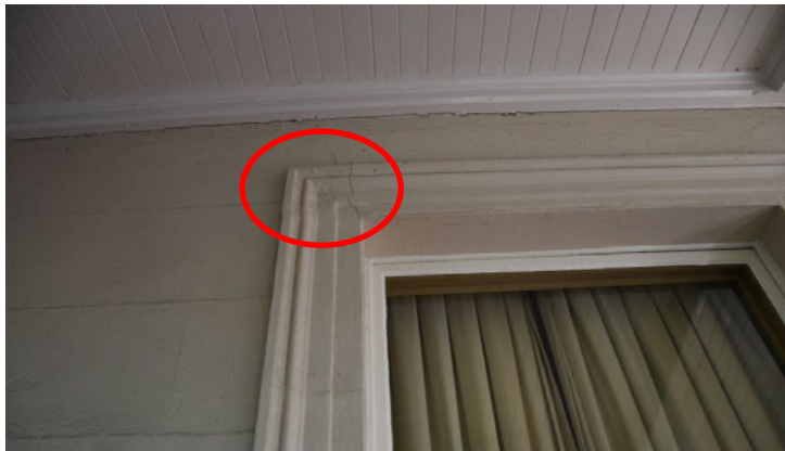
Figure 11 Hairline crack reportedly caused by the Ficus macrocarpa.
