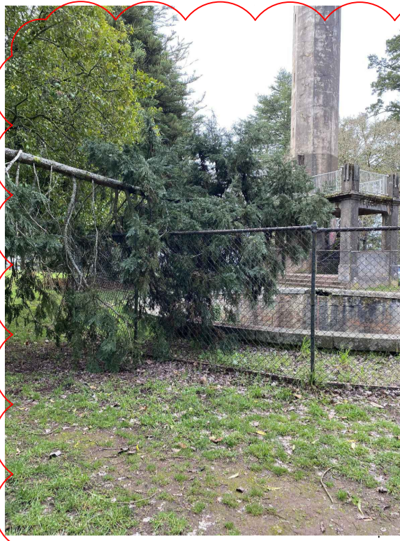
Overhanging tree branch to be removed
