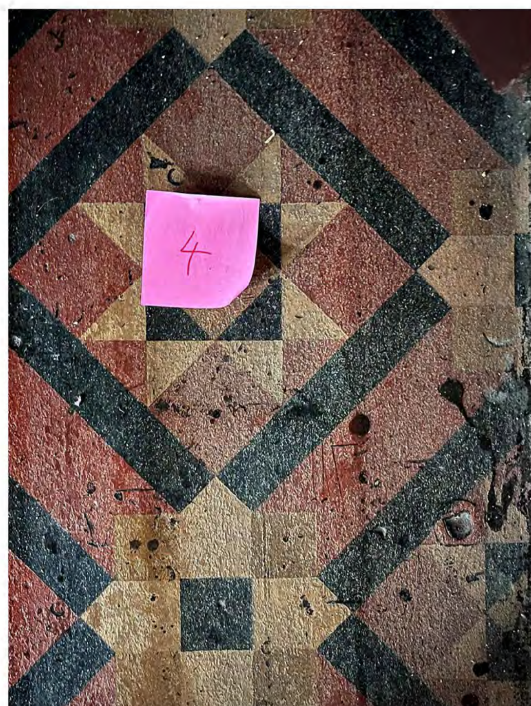
CODE: 3 CONDITION RATING: VERY POOR NUMBER: 4 GRID LOCATION: 3-GG
