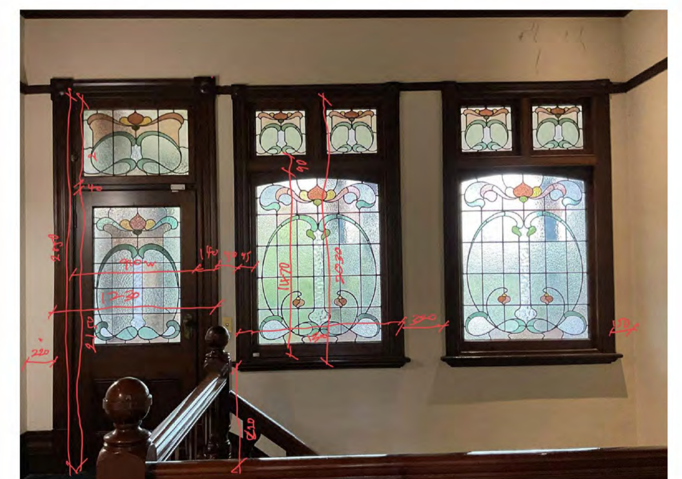
W1.01 W1.02 W1.03 AREAS OF NON-ORIGINAL GLAZING TOP LITES HAVE SIGNS OF BOWING
