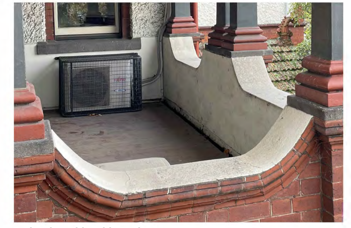
EXISTING BALCONY CONDITION EXISTING BALCONY CONDITION HAS FOLLOWING NON-COMPLIANCES AND RESTORATION WORKS REQUIRED: - NON-COMPLIANT LOW BALUSTRADE - REQUIRES DISPENSATION. - DRAINAGE SLOT NOT IN WORKING ORDER. - BOTH DRAINAGE SLOT AND BALCONY LEAKING TO PORCH BELOW.
