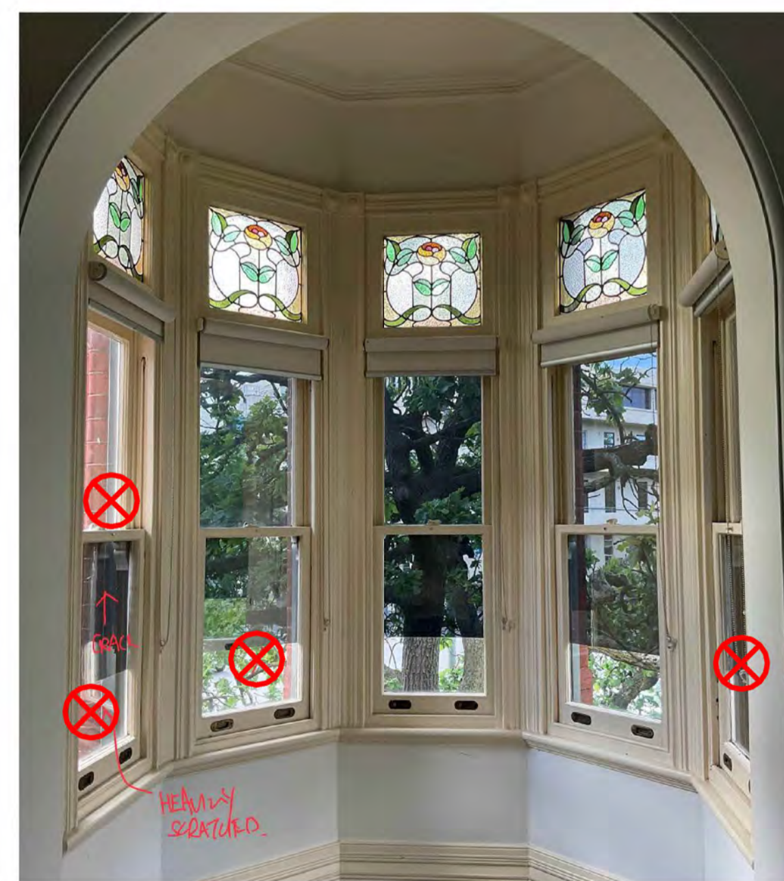
W1.04 W1.05 W1.06 W1.07 W1.08 TOPLIGHTS HAVE SIGNS OF BOWING
