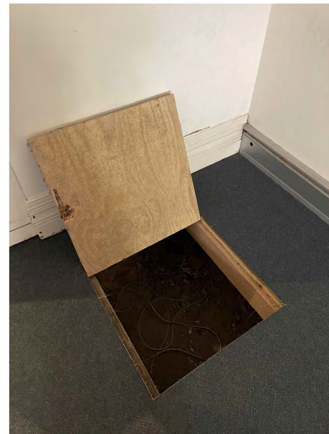
EXISTING CARPET OVER NON-ORIGNAL PLYWOOD FLOOR
