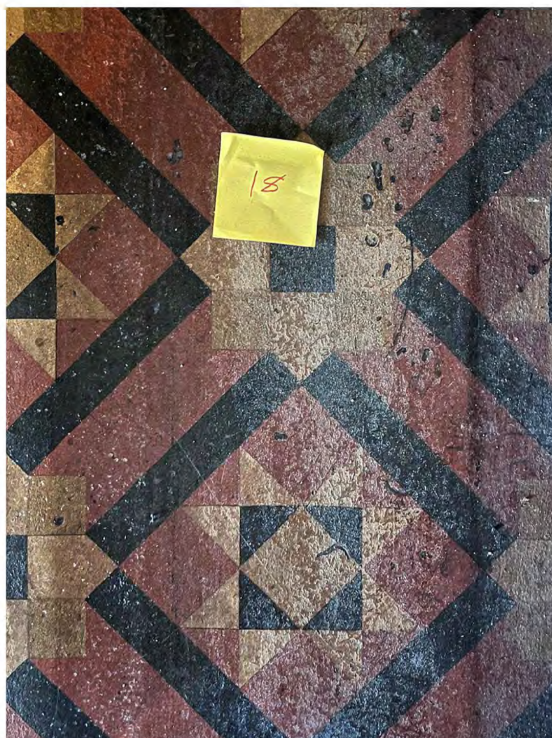
CODE: 2 CONDITION RATING: POOR NUMBER: 18 GRID LOCATION: 3-EE
