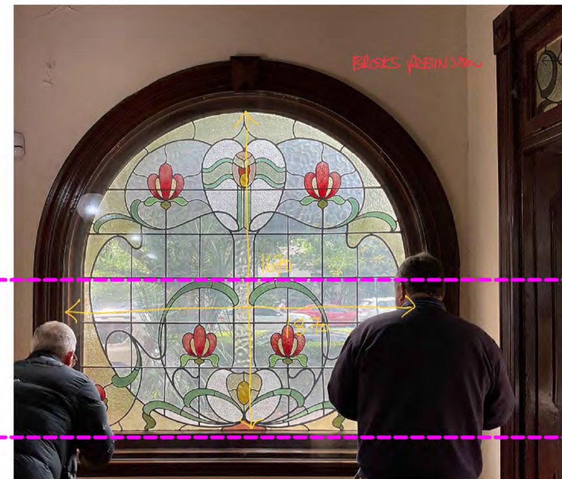
WG.01 STAINED GLASS - HEAVY BOWING WILL REQUIRE REPAIR OFF-SITE
