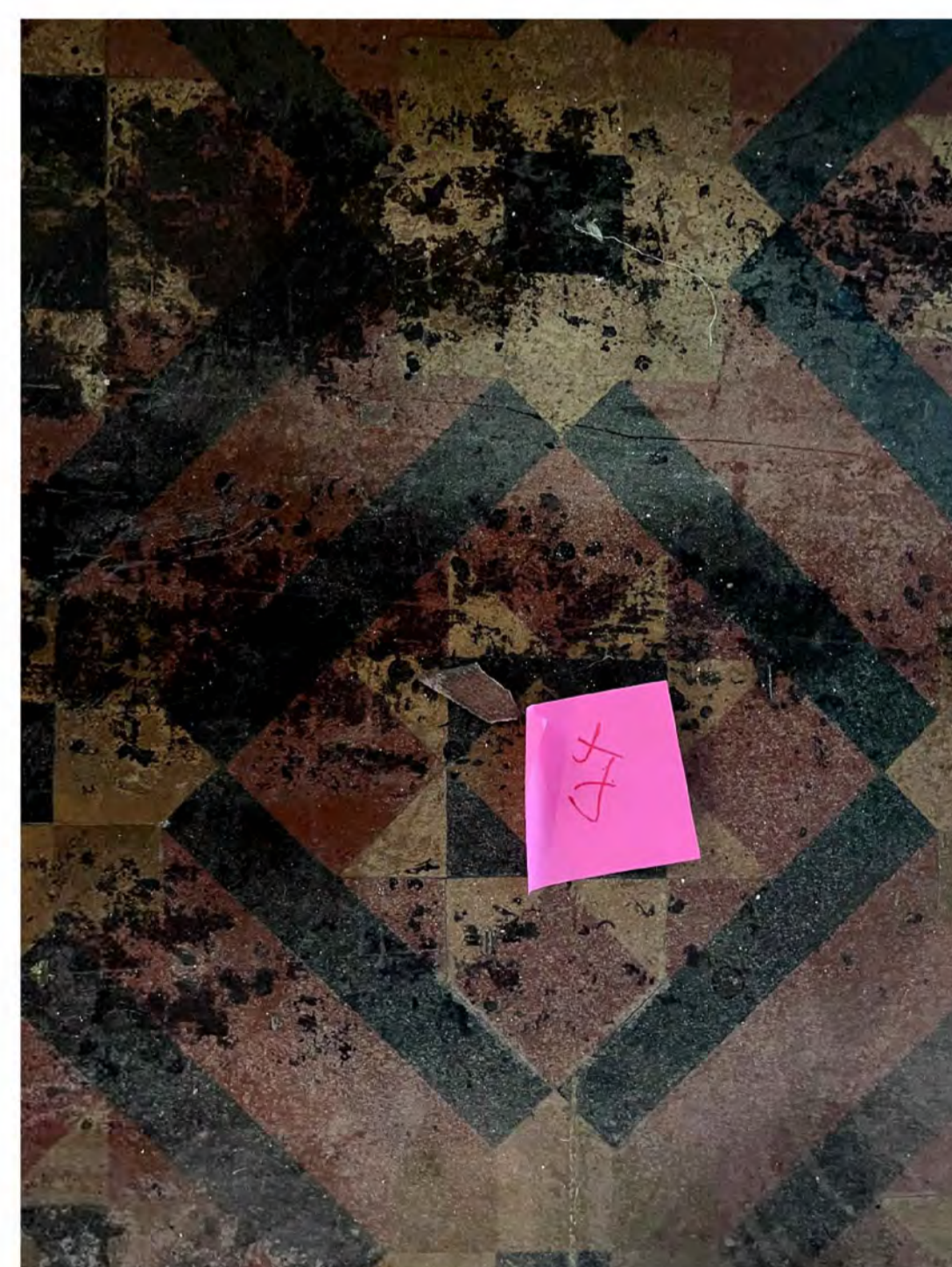
CODE: 3 CONDITION RATING: VERY POOR NUMBER: 44 GRID LOCATION: 5-AA
