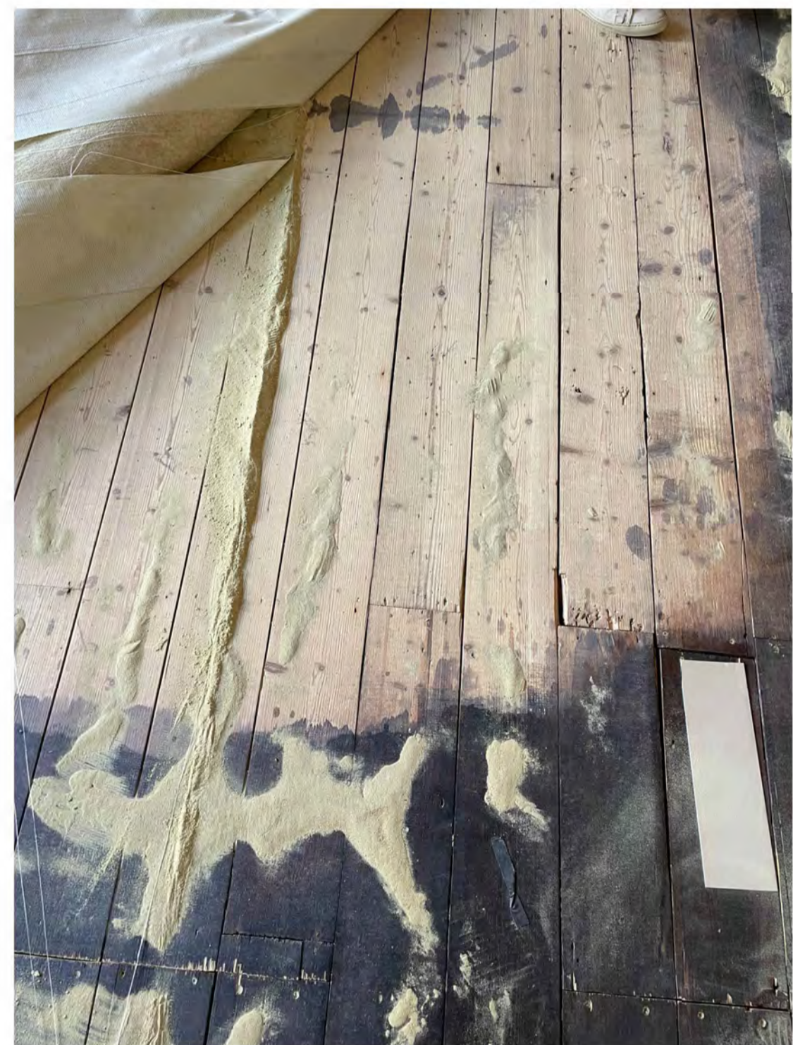
EXISTING BALTIC PINE FLOORBOARDS DISCOLORATION & QUALITY REFERENCE
