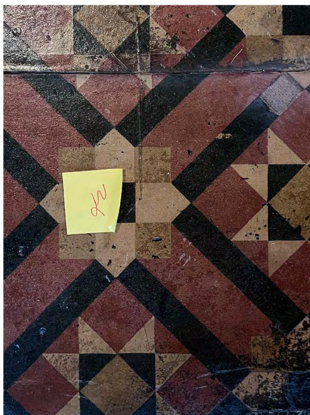
CODE: 2 CONDITION RATING: POOR NUMBER: 36 GRID LOCATION: 4-BB
