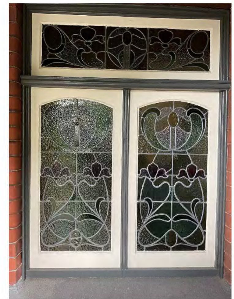
WG.03 STAINED GLASS - HAVE NON-ORIGINAL GLASS PANELS AND CRACKS FIXED OVER TIME
