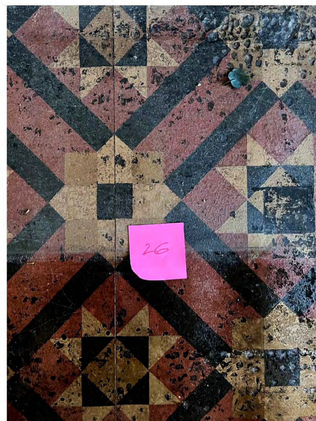
CODE: 3 CONDITION RATING: VERY POOR NUMBER: 26 GRID LOCATION: 5-DD
