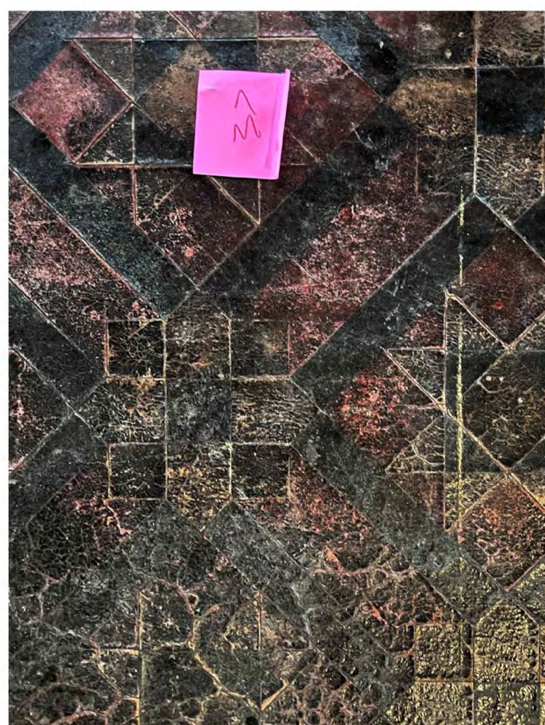
CODE: 3 CONDITION RATING: VERY POOR NUMBER: 37 GRID LOCATION: 5-BB
