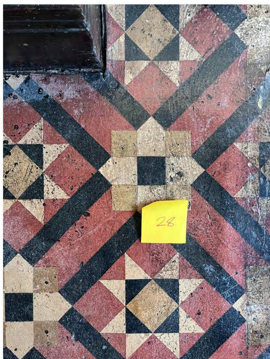
CODE: 2 CONDITION RATING: POOR NUMBER: 28 GRID LOCATION: 6-DD
