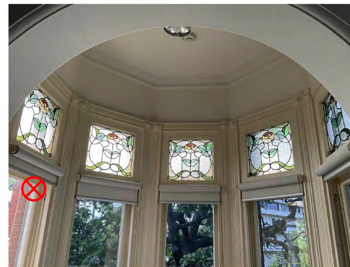
WG.04 WG.05 WG.06 WG.07 WG.08 STAINED GLASS TOPLIGHTS - ALL BOWING, BUT OTHERWISE IN GOOD CONDITION
