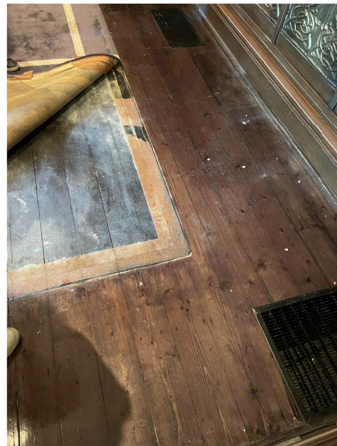
EXISTING BALTIC PINE FLOORBOARDS DISCOLORATION & QUALITY REFERENCE
