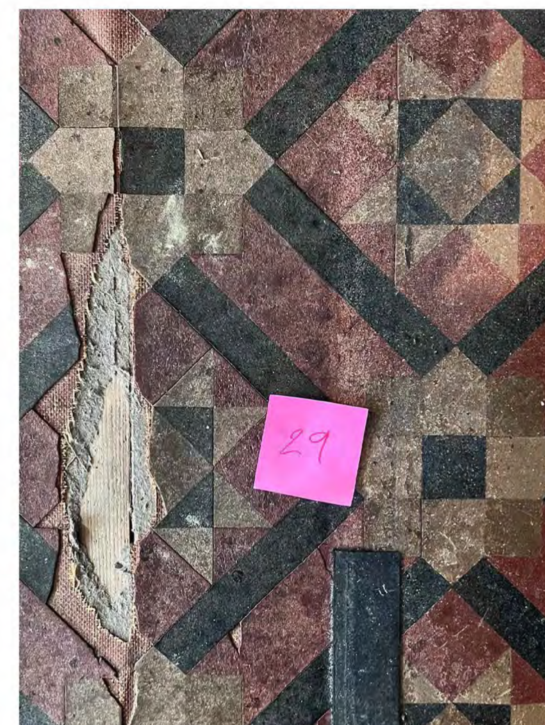
CODE: 3 CONDITION RATING: VERY POOR NUMBER: 29 GRID LOCATION: 2-CC
