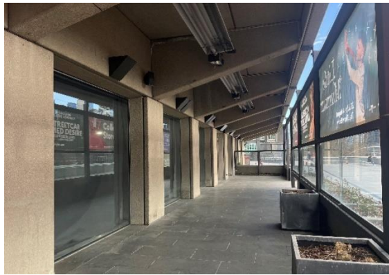
Figure 22 West end of the project area, note later steel structure with glazing and planter boxes partially enclosing the exterior walkway. Source: Trethowan Architecture, 2024.
