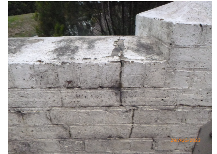
DEFECT 10: CRACKS ON TOP FACE OF WEST END SOUTHERN PARAPET
