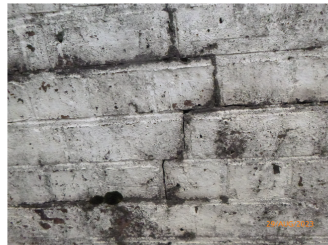
DEFECT 3: CRACKS PROPAGATING OVER 4NO. BRICKS AT WEST END OF NORTHERN PARAPET
