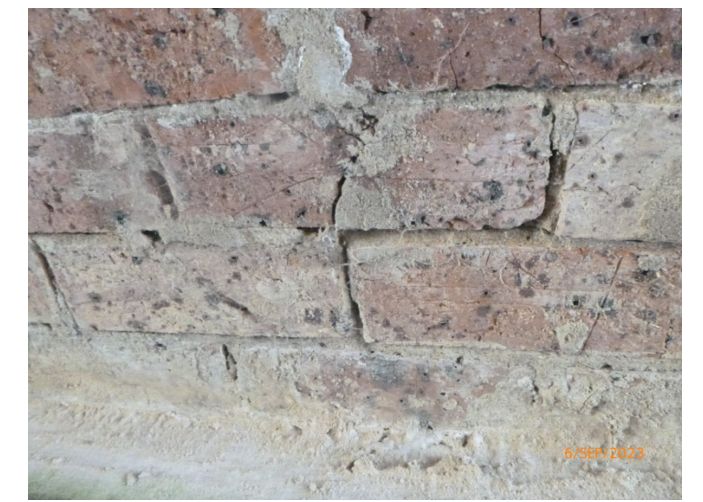
DEFECT 20: MORTAR LOSS ON TWO LAYERS OF BRICKS ABOVE EAST WATERWAY INVERT PROTECTION
