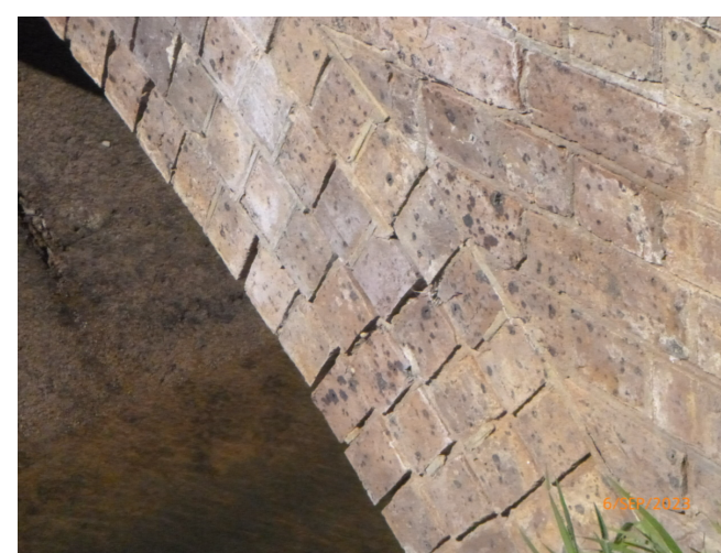
DEFECT 16: MORTAR LOSS ON NORTHERN FACE OF ARCH RING
