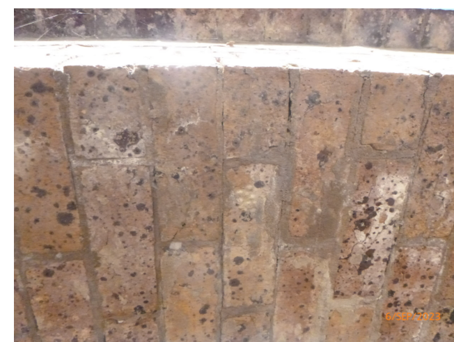
DEFECT 19: FULL LENGTH TRANSVERSE CRACK ACROSS ENTIRE LENGTH OF ARCH CROWN
