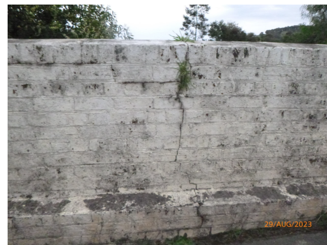
DEFECT 8: FULL HEIGHT CRACK CLOSE TO EAST END OF SOUTHERN PARAPET
