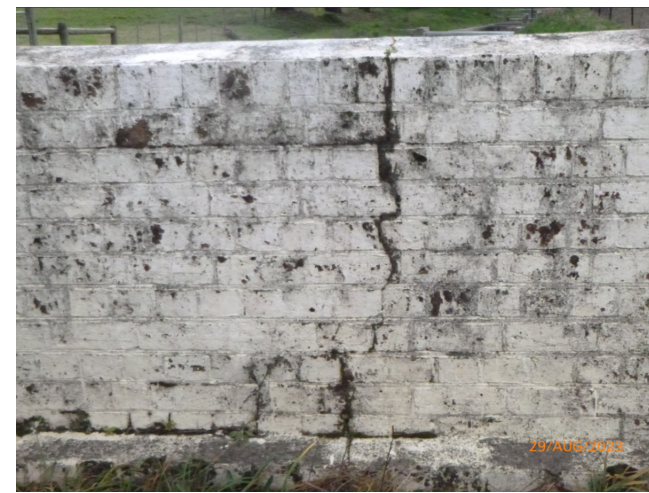
DEFECT 4: FULL HEIGHT CRACK AT MIDSPAN OF NORTHERN PARAPET
