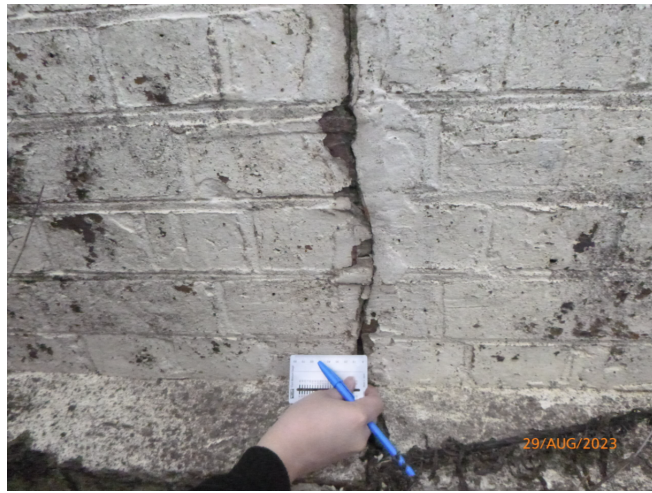
DEFECT 2: FULL HEIGHT CRACK CLOSE TO EAST END OF NORTHERN PARAPET
