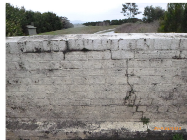
DEFECT 9: FULL HEIGHT CRACK AT MIDSPAN OF SOUTHERN PARAPET
