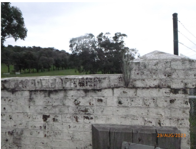
DEFECT 7: HORIZONTAL CRACK ALONG TOP LAYER OF BRICK AT NORTHERN PARAPET
