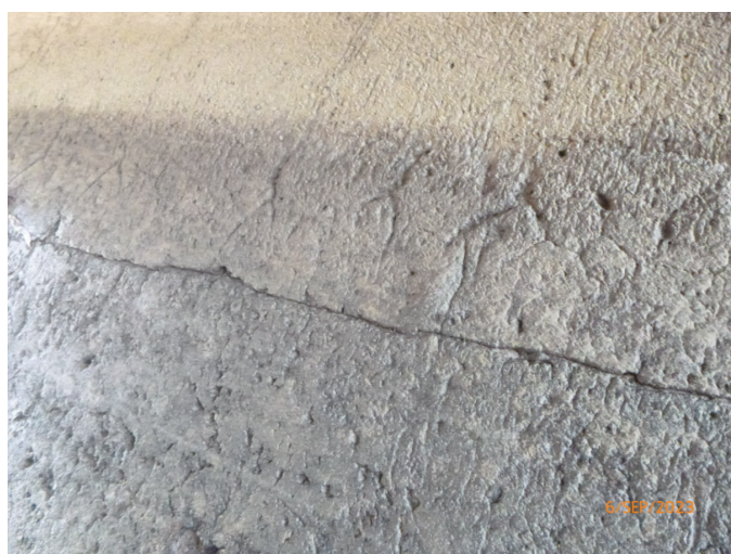
DEFECT 13: FULL LENGTH LONGITUDINAL CRACK ACROSS EAST WATERWAY INVERT PROTECTION FACE
