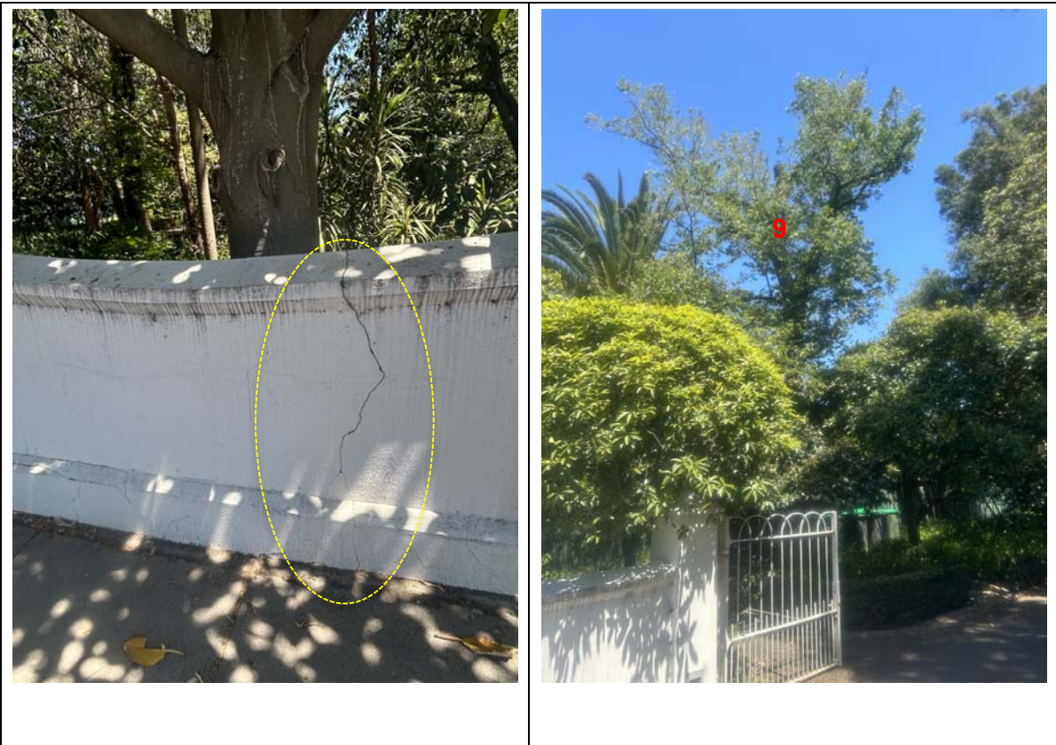
Figure 9 (above left): Shows cracking to the front boundary fence from the roots of Tree 17.
