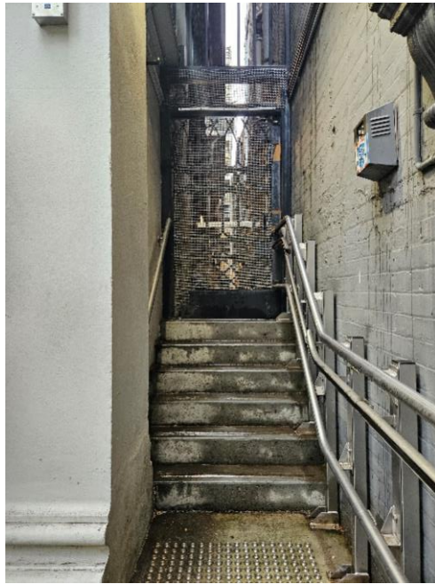
Figure 27: Image of the area to the southeastern corner showing the concrete stairs from the topmost platform to the breezeway.
