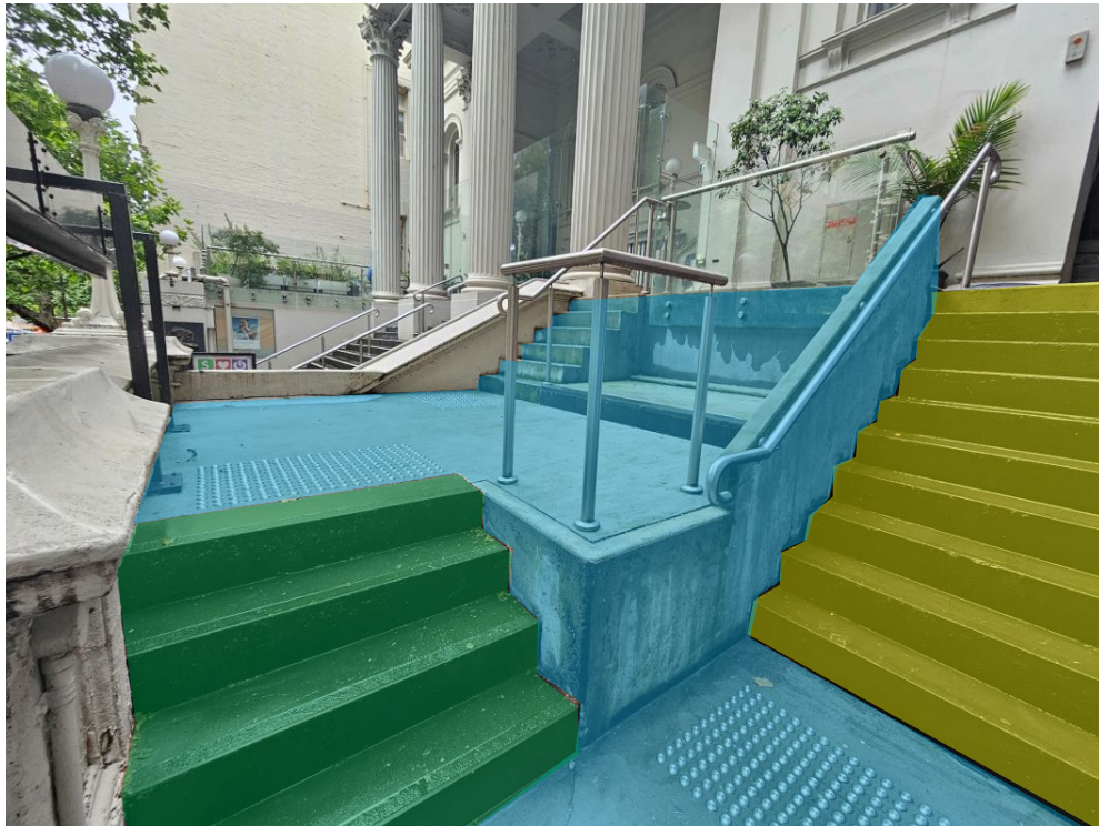
Figure 33: The fabric shaded blue was introduced to this area in 2010. The smaller of the bluestone stairs shaded green was introduced at this time and constructed from new and remodelled existing bluestone, possibly from the porch. The bluestone stairs shaded yellow were considerably modified in 2010 when new bluestone raisers were created from the former bluestone steps; new bluestone was also introduced.
