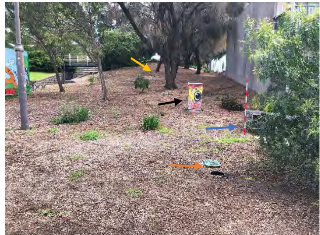
Photograph 11 Multiple underground assets; water (yellow), telecommunications (black), electricity (orange), gas (blue). North east corner, facing west (W. Hernandez 13/10/2023)
