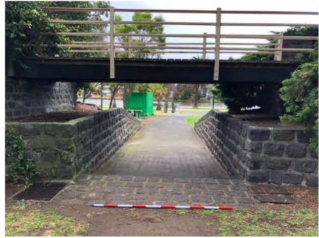
Photograph 13 Drainages, bluestone pavement and bitumen footpath under the pedestrian bridge, taken from the northern exit point of the amphitheatre (W. Hernandez 13/10/2023)
