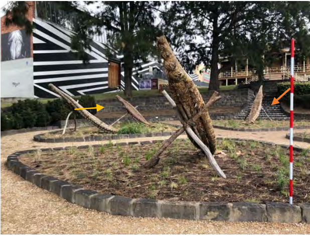
Photograph 12 Retaining walls (yellow), garden beds, access stairs (orange), facing south west (W. Hernandez 13/10/2023)
