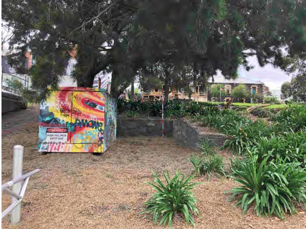
Photograph 8 High voltage electricity, south west corner, facing west (W. Hernandez 13/10/2023)
