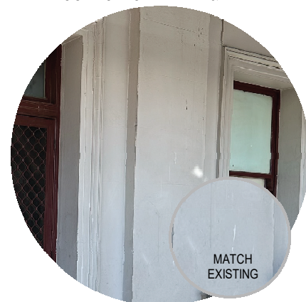
EXISTING WALL COLOUR: TO MATCH EXISTING SOUTH STATION BUILDING LOCATION: SOUTH BUILDING
