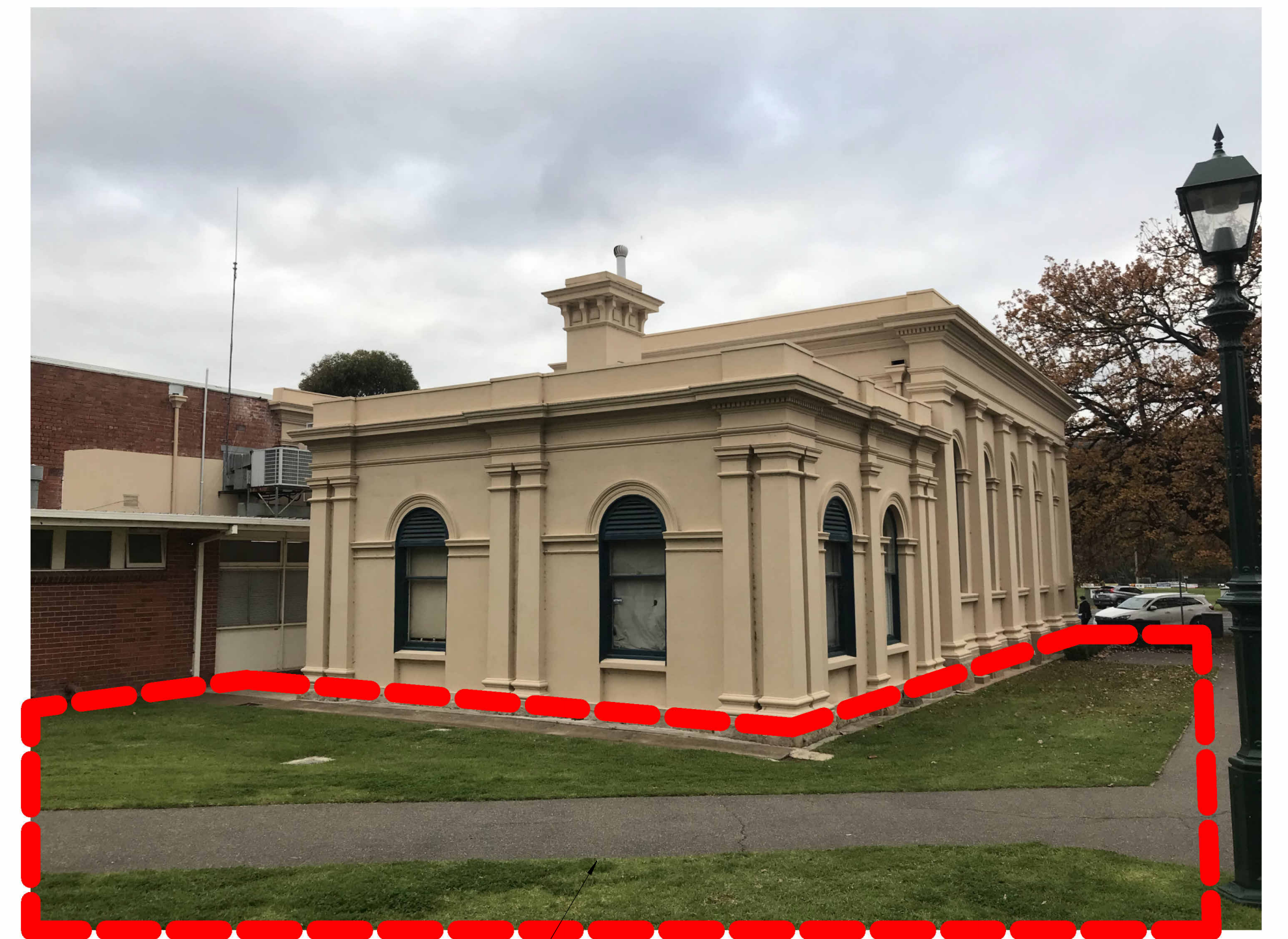
Excavate down to exposed existing courthouse building floor vent (approx -300mm). Modified land contour to match back in to existing
