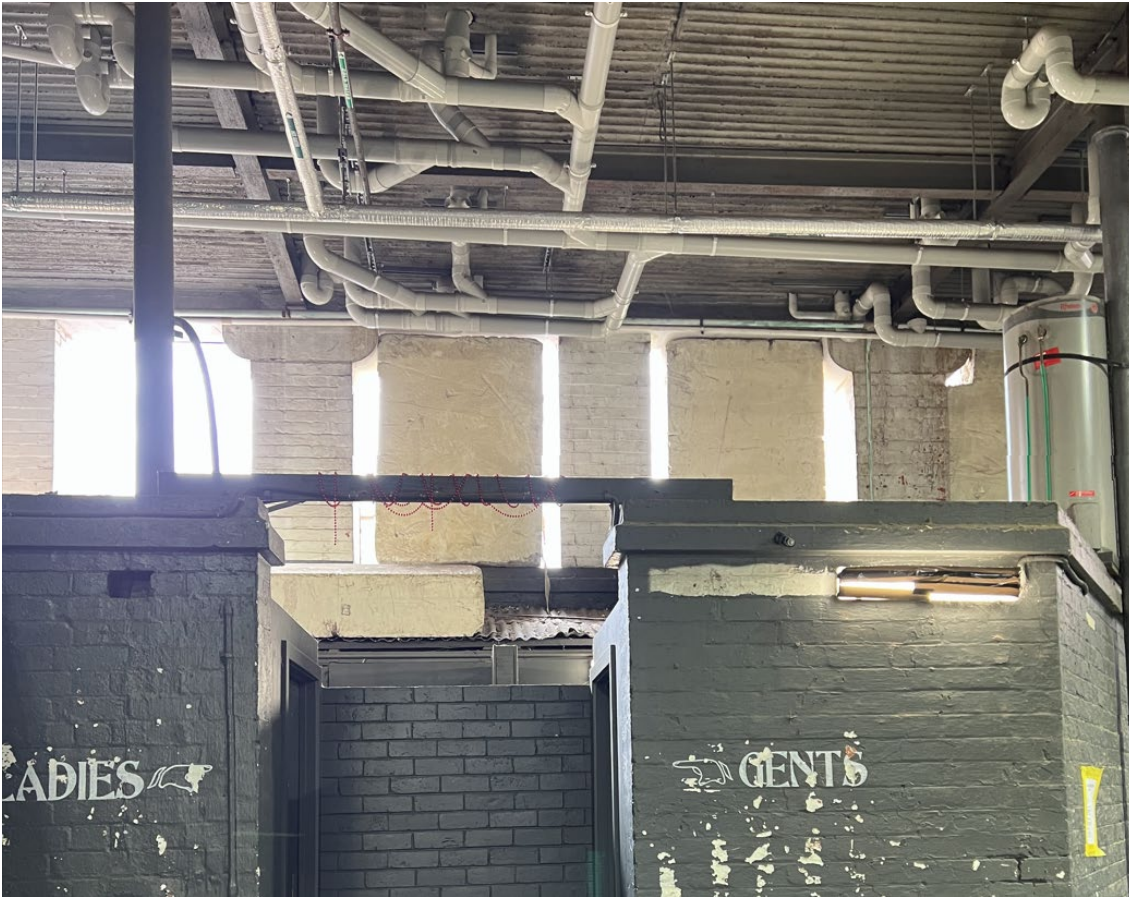
Figure 15 Openings on east wall above undercroft toilets with unfixed polystyrene infills proposed for removal
