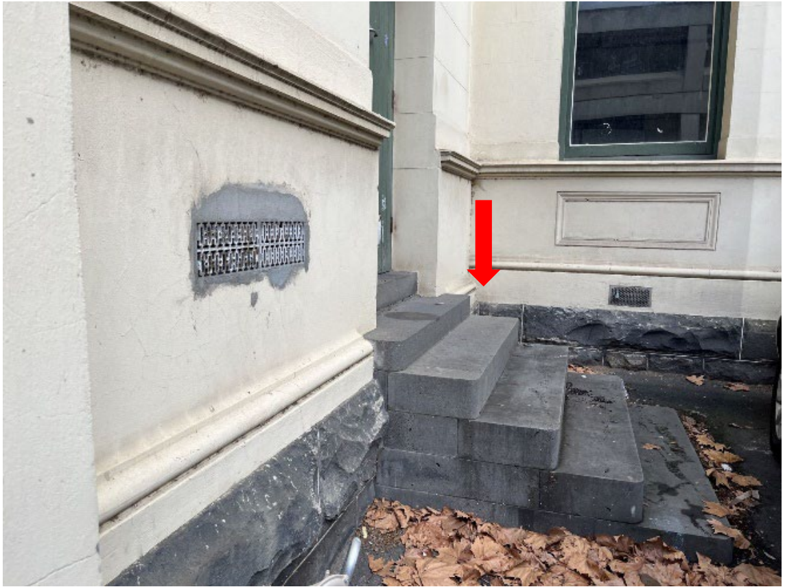
Figure 19 Non-original bluestone stairs in carpark north of Stage 9, to be dismantled and reconstructed in a new arrangement with new landing and integrated handrails
