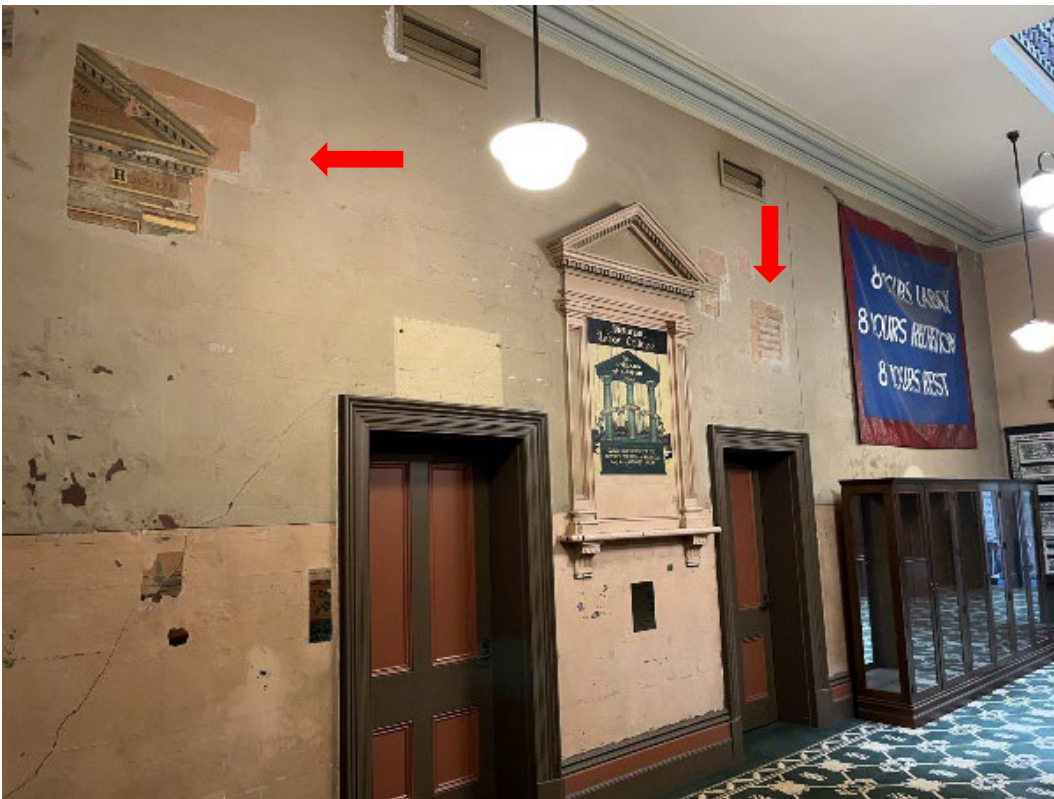
Figure 8 Revealed sections (indicated) of overpainted honour rolls on west wall of entry hall (G46)
