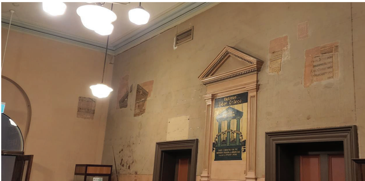
Figure 13 Overview of the paint removal trial areas on the south and west walls.
