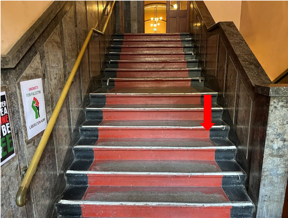
Figure 17 Ground level entry stairs to Victoria Street wing showing location of proposed handrail to be fixed to concrete floor
