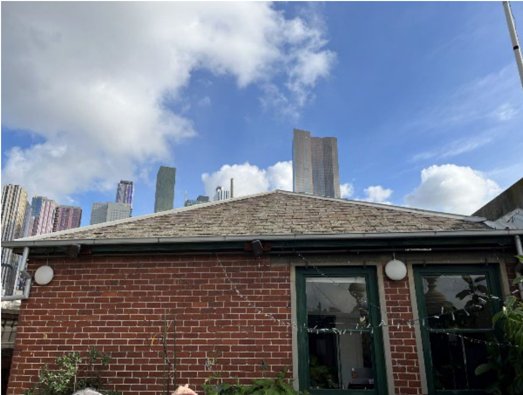
Figure 11 Slate clad roof of the Caretaker's Cottage showing existing ridge capping, gutters and downpipes to be demolished
