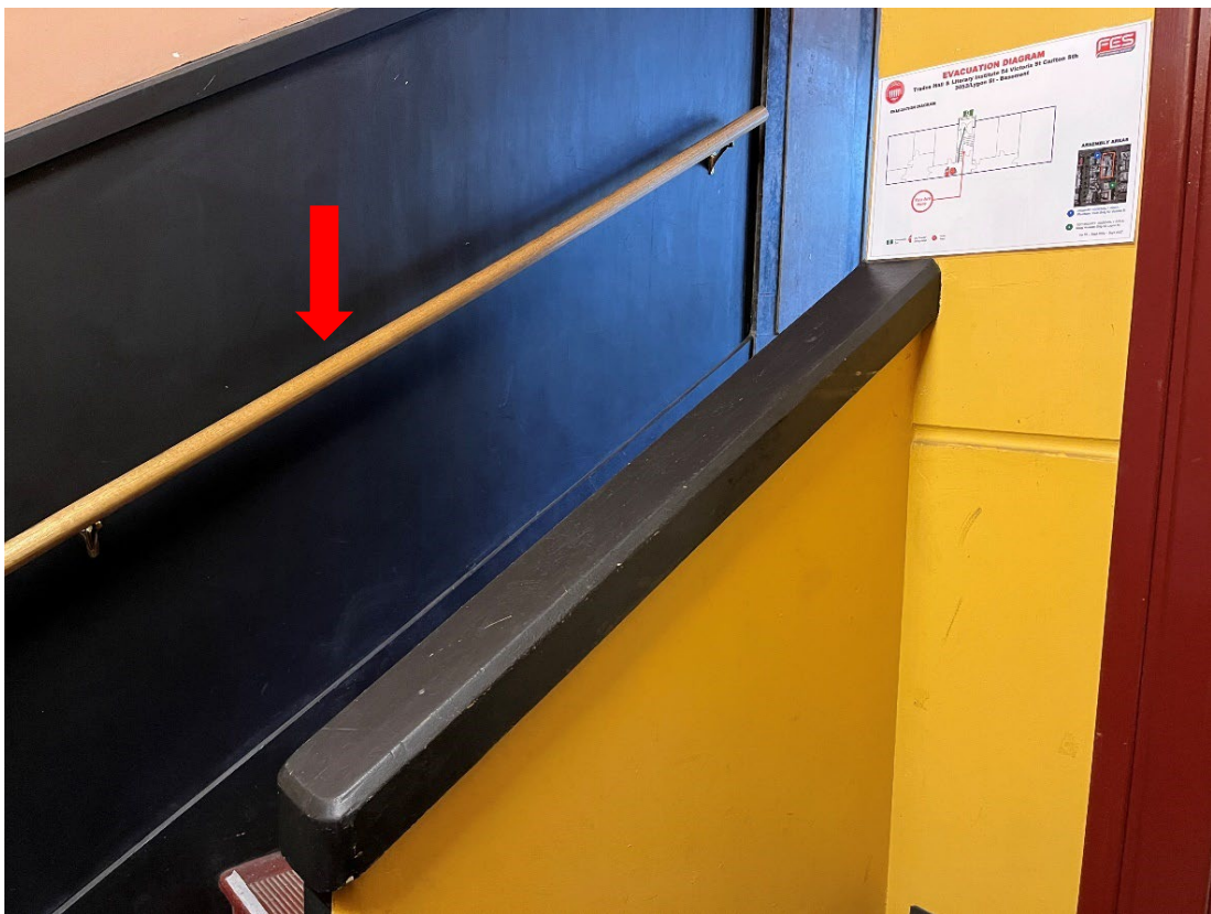
Figure 16 Stairs to basement from Victoria Street entry showing non-original timber handrail proposed for removal
