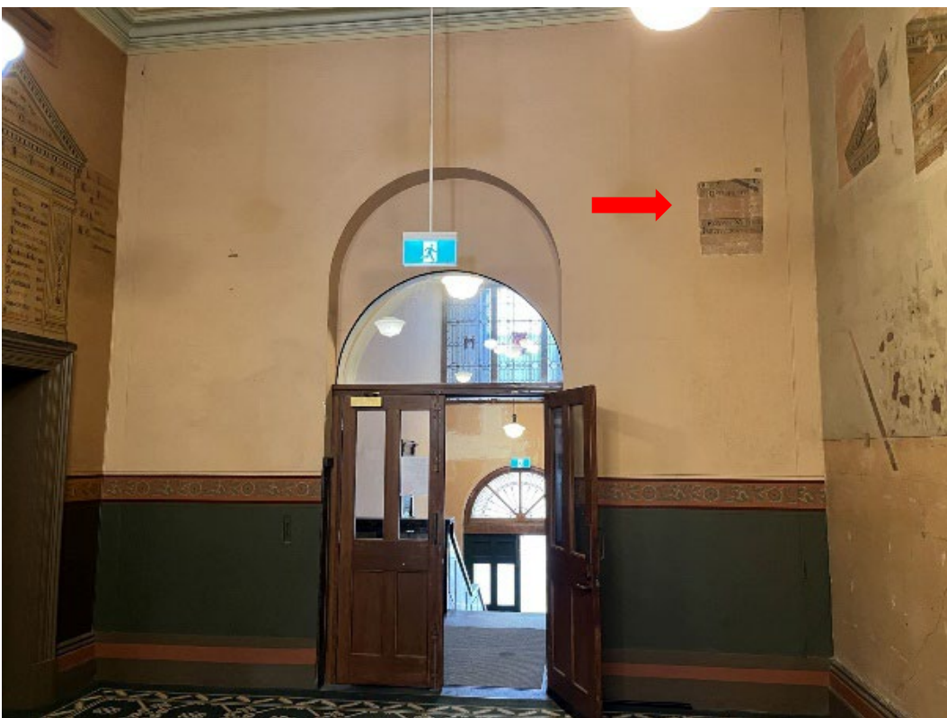
Figure 9 Revealed section (indicated) of overpainted honour roll on south wall of entry hall (G46)
