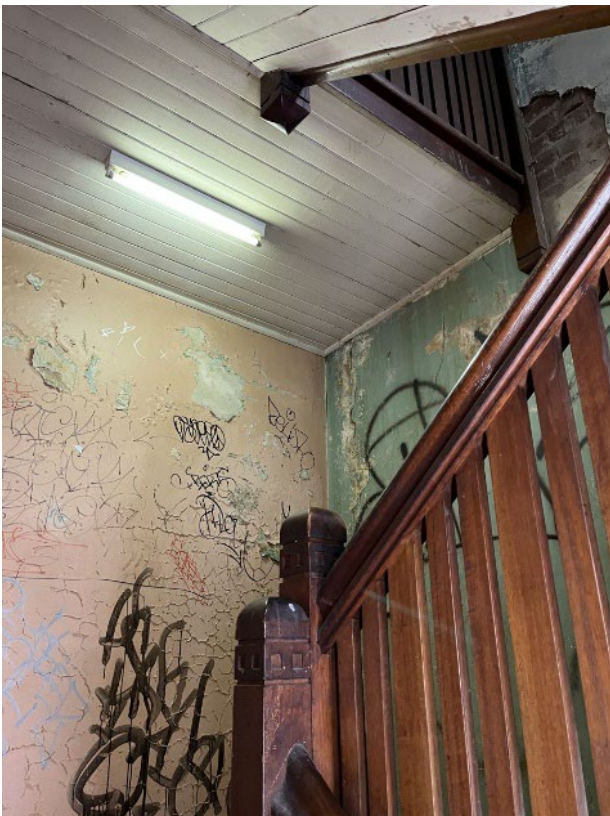
Figure 18 Typical condition found in Stair 2, north-east corner of Stage 9
