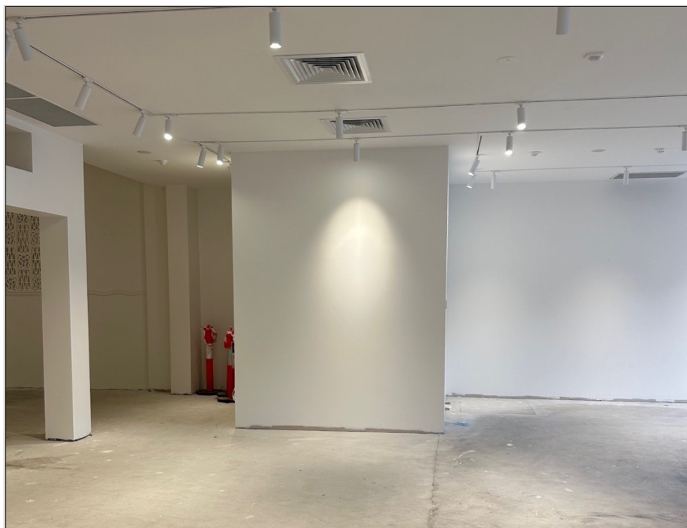
Figure 13 Current photograph of the foyer showing the stairs enclosed in a stud wall.
