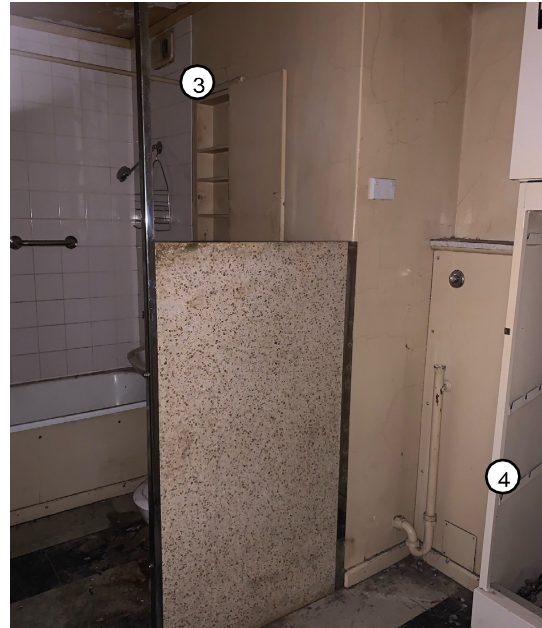
January 2022, 20 Elgin Street, bathroom of an apartment. Source: Homes Victoria.
