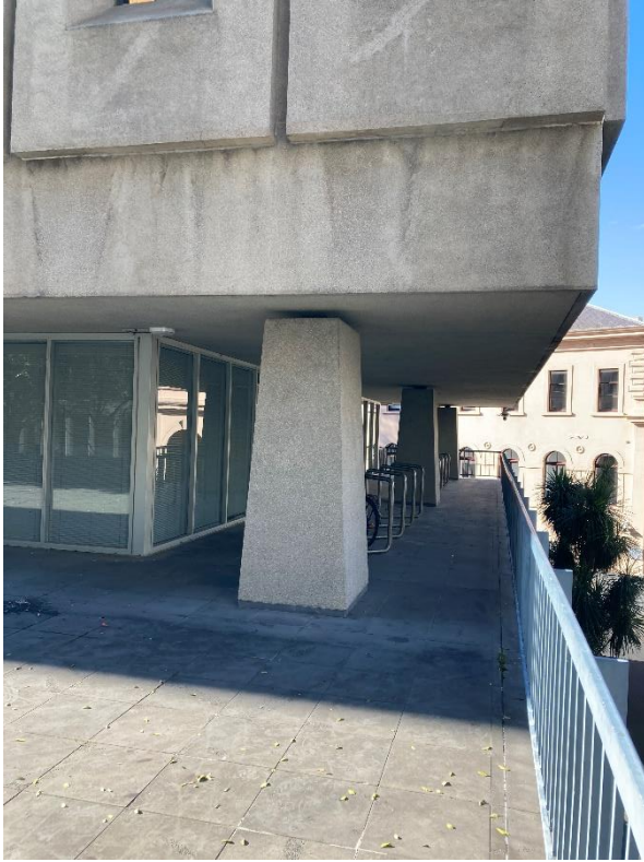
Figure 9 View east along the ground floor to the south of the building
