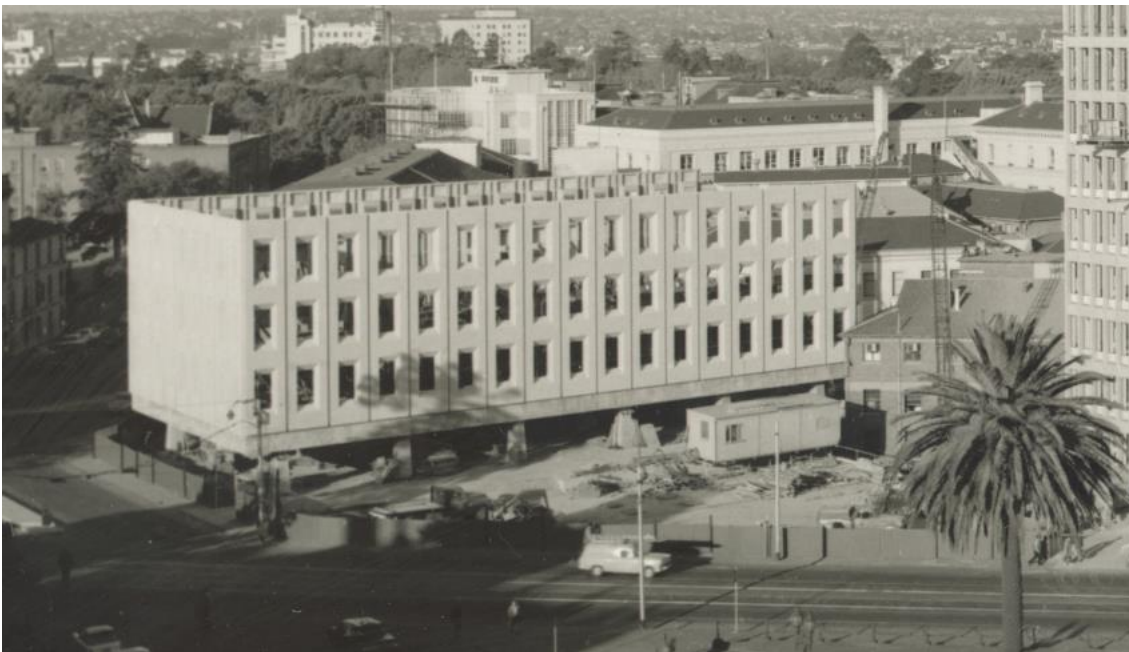
Figure 4 1967 image of the subject building under construction, prior to the addition of the upper level in 1996
