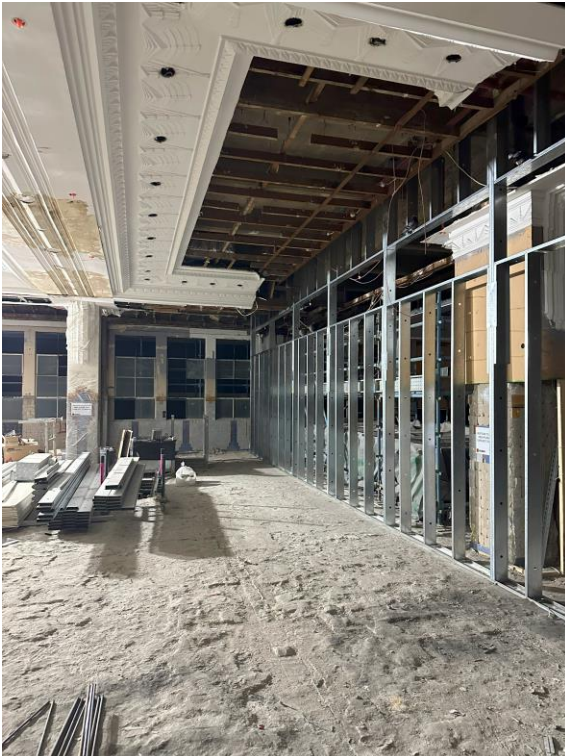
First floor level – full height inter-tenancy wall approved under base build permit (P34021)
