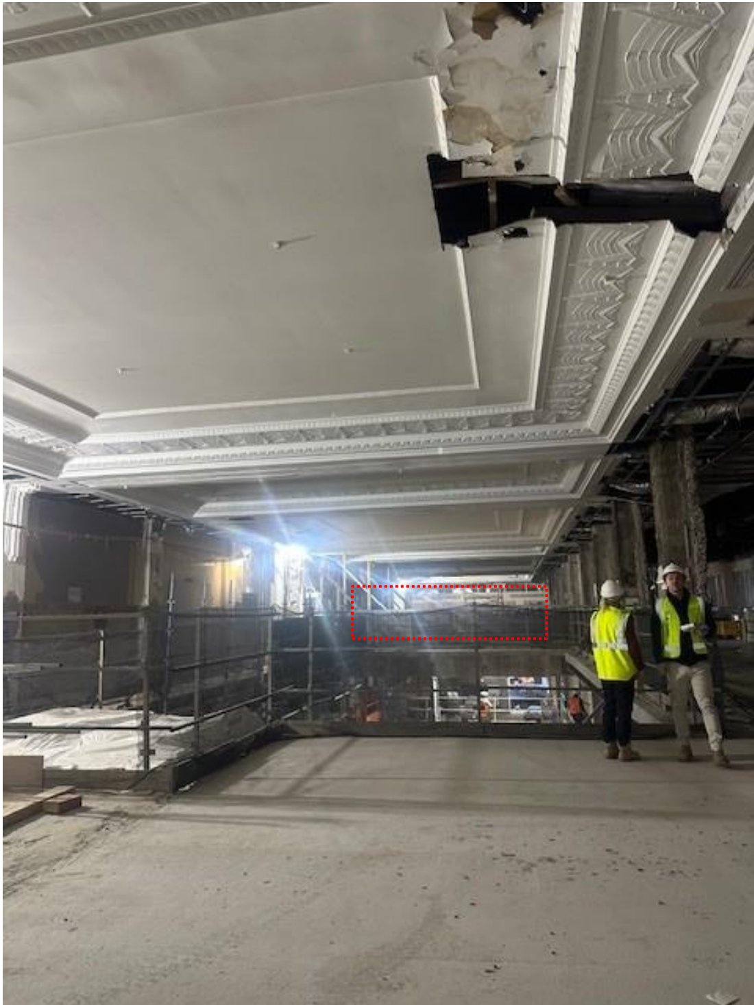
View from first floor level, looking south across the void towards the location of the proposed Meccaversity (photo courtesy of MECCA)
