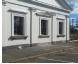
Reconstructed bay to the west end of the north side of station building refer P20705
