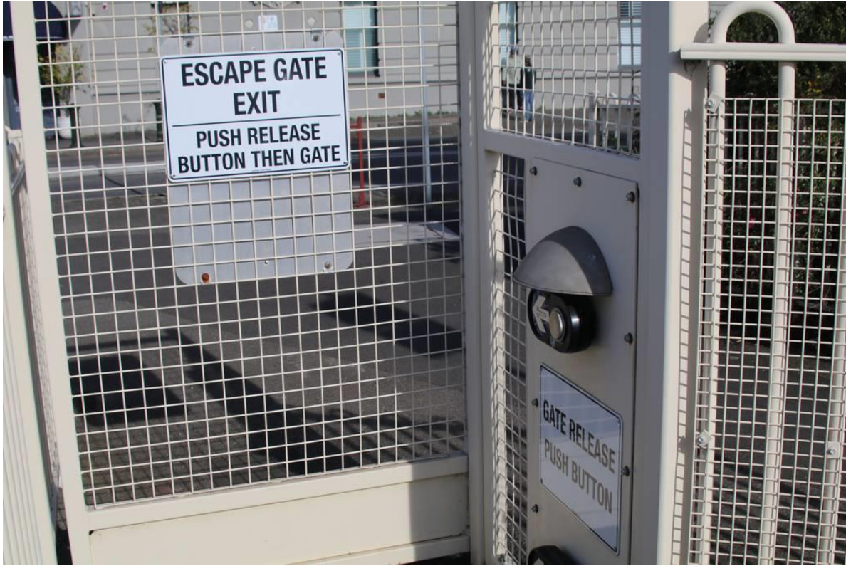
Figure 8 Emergency egress gate latch release
