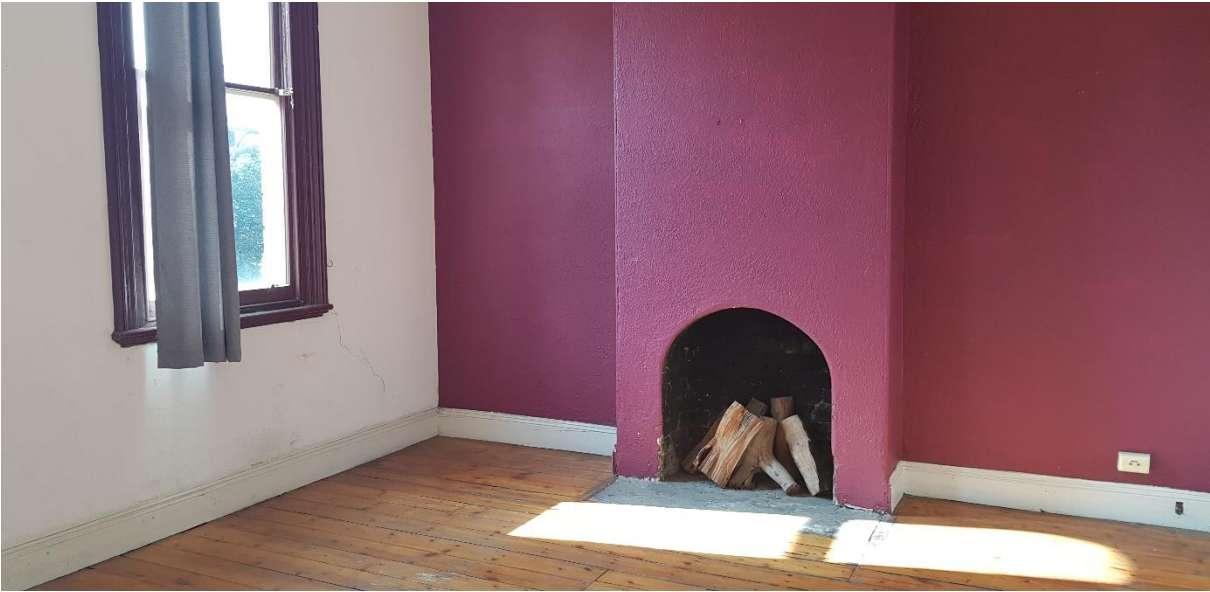
Figure 23 Master bedroom showing fireplace with missing mantelpiece
