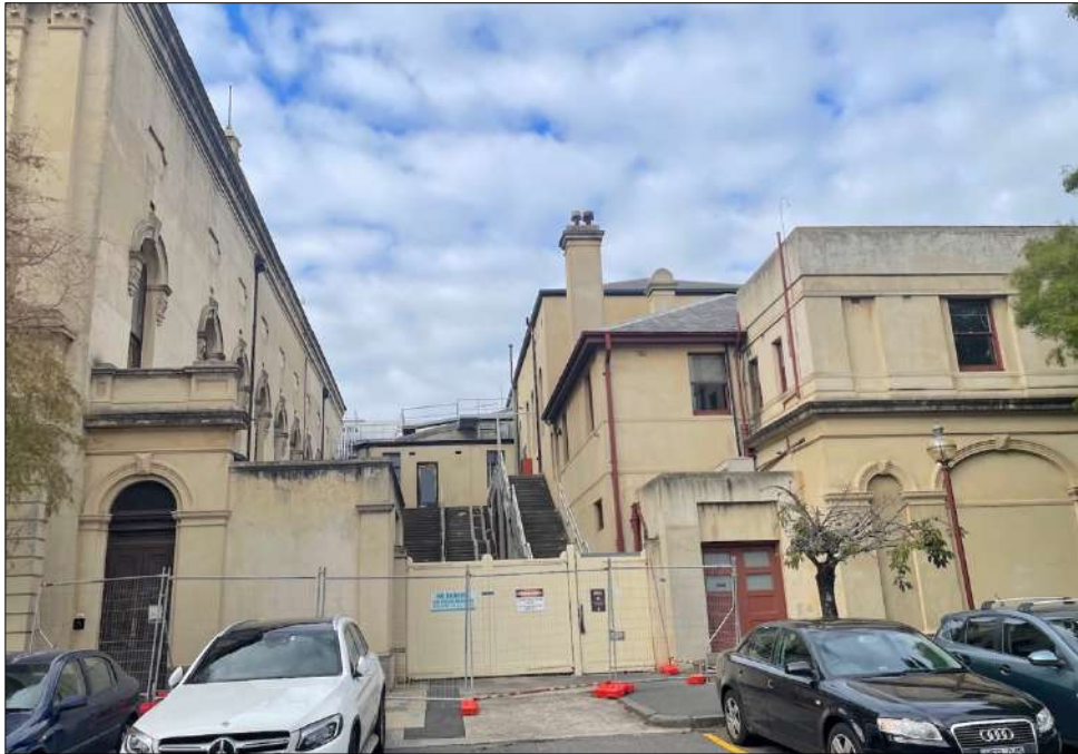
Figure 23 The north elevation showing the service courtyard and c1936 first floor assistant librarian's flat (top right).
