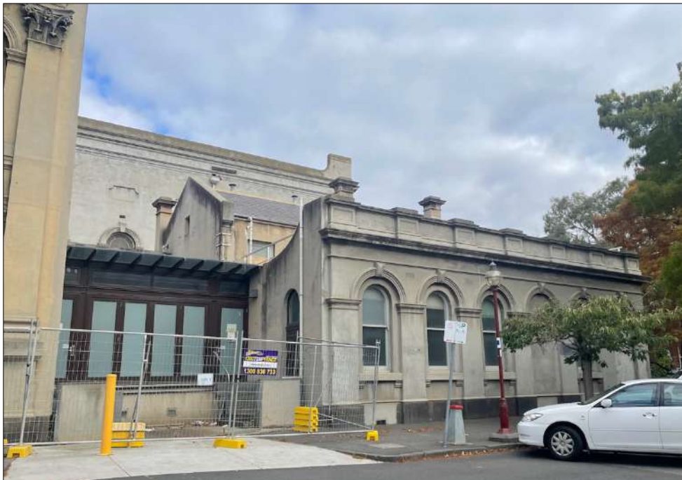
Figure 20 The northern end of the east elevation showing the 1990s loading bay/infill (left) and former courthouse (right).
