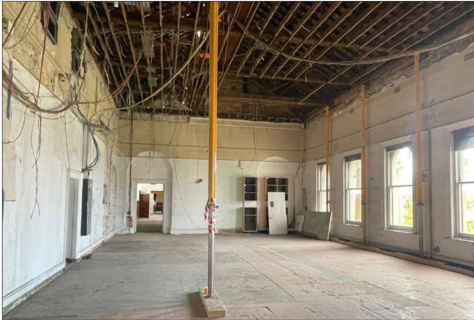
Figure 33 The former supper room on the first floor of the front wing.
