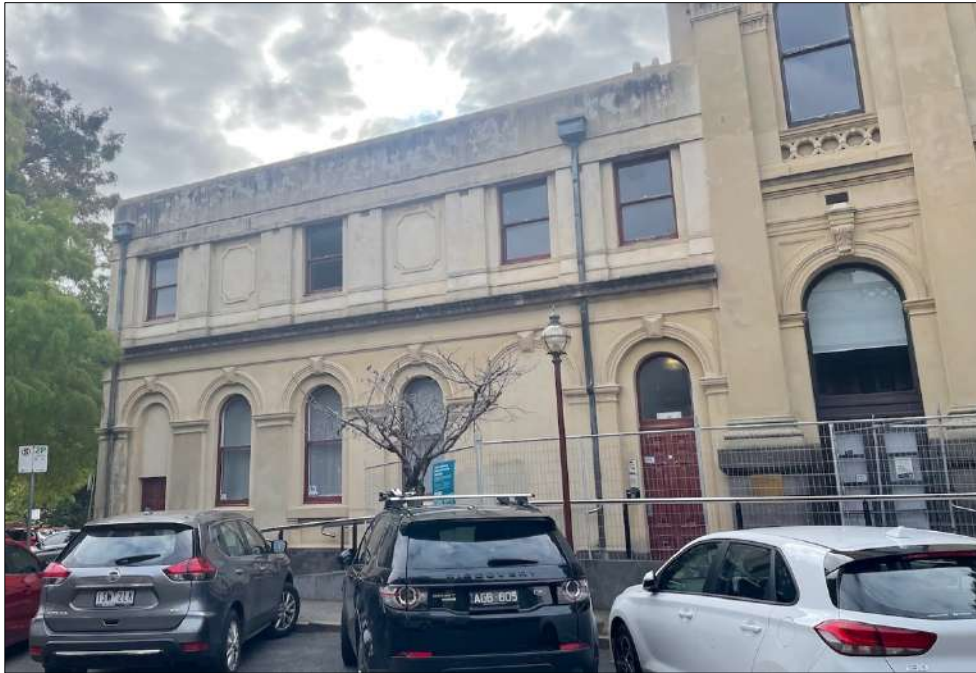
Figure 25 Partial view of the west elevation showing the c1936 first floor addition (former assistant librarian's flat).
