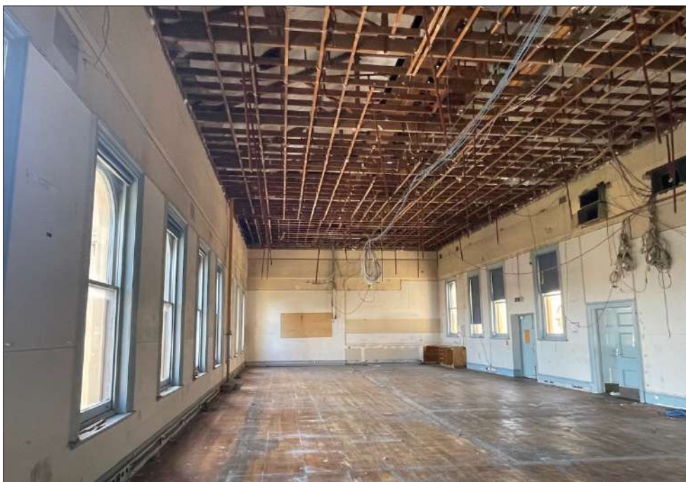
Figure 34 Former Mechanics' Institute lodge room, first floor of the west wing. The ceiling was removed in recent years to allow for the condition of the roof trusses to be investigated.
