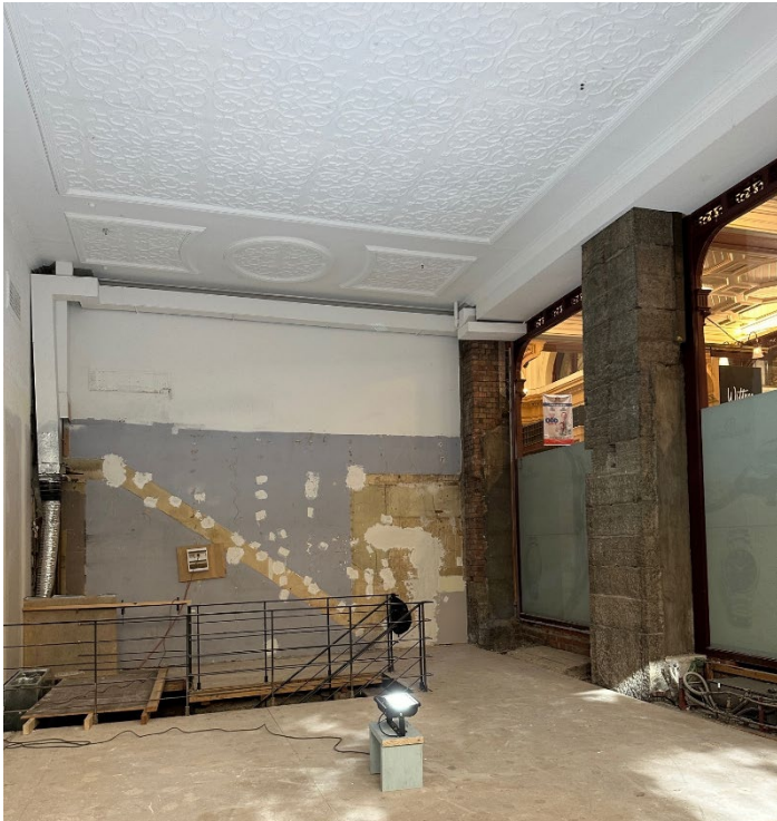
Figure 6 View of the tenancy showing the division of the space post Kodak's rental.
