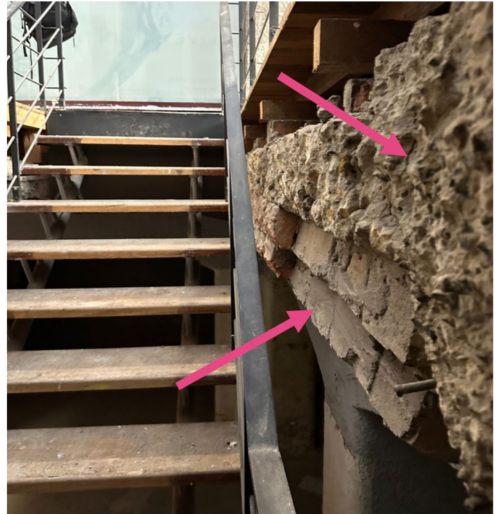
Figure 10 Existing stair opening showing remnant brick vault and chunk of infill concrete proposed to be removed to accommodate new stair.
