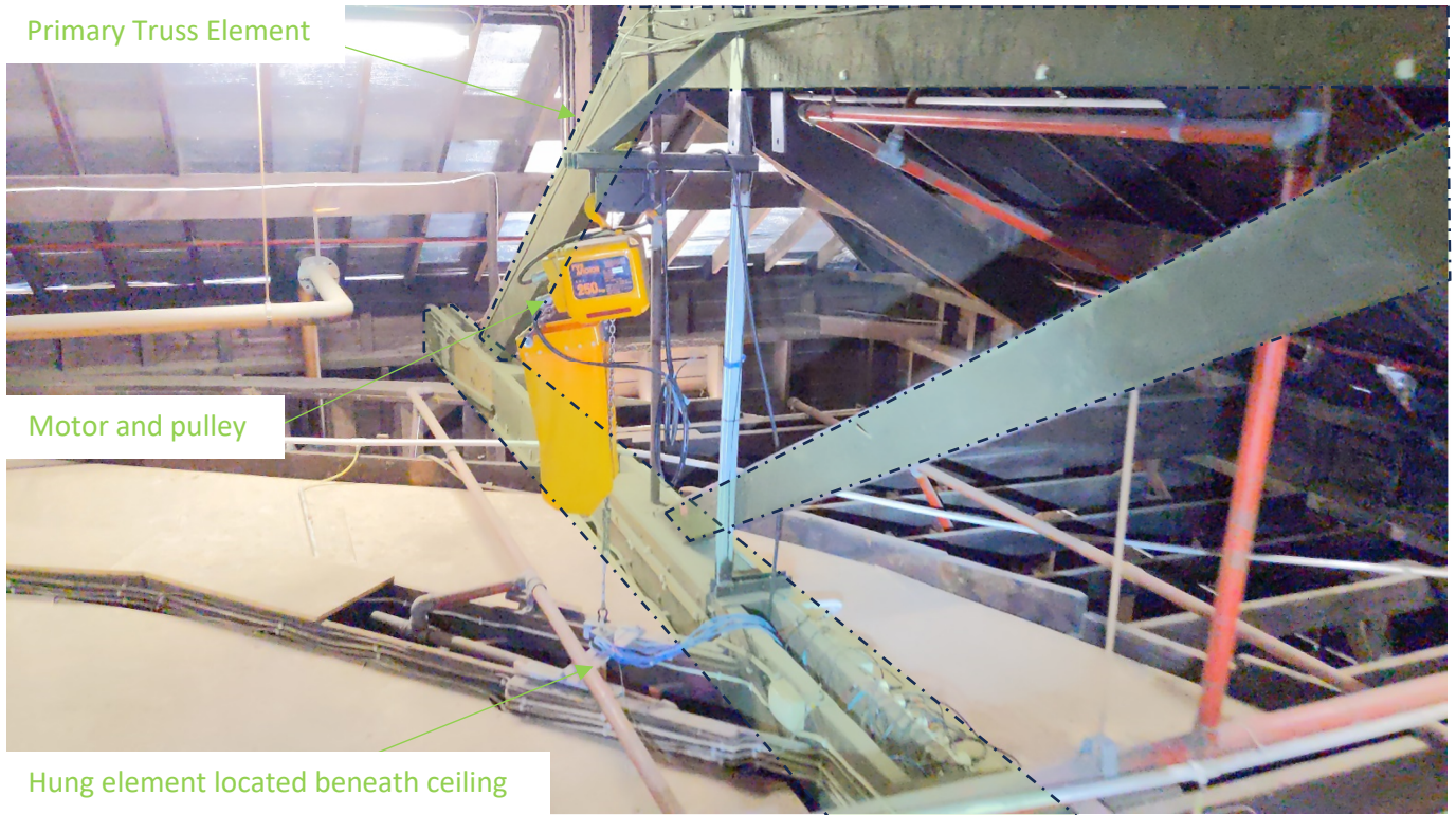
Figure 6 – Photo taken within the ceiling space identifying primary support truss and hung element attached directly to the primary truss.
