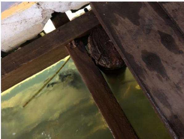
The structure has dropped at the rear (North Eastern corner).
