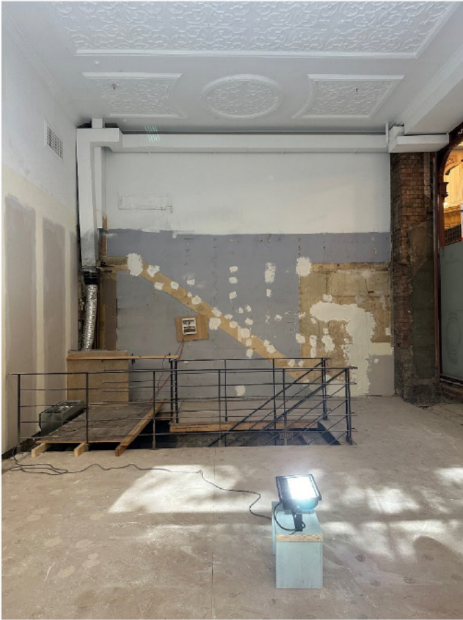
Figure 1 View of the interior of the subject site showing the shadow of a former stair stringer on the end wall where the mezzanine is proposed to be installed.
