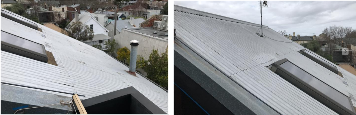
More views of the south elevation roof - note cut out sections for skylights and therefore limited roof slope on this elevation, also south is the least satisfactory location for solar panels due to limited sun access in Melbourne.
