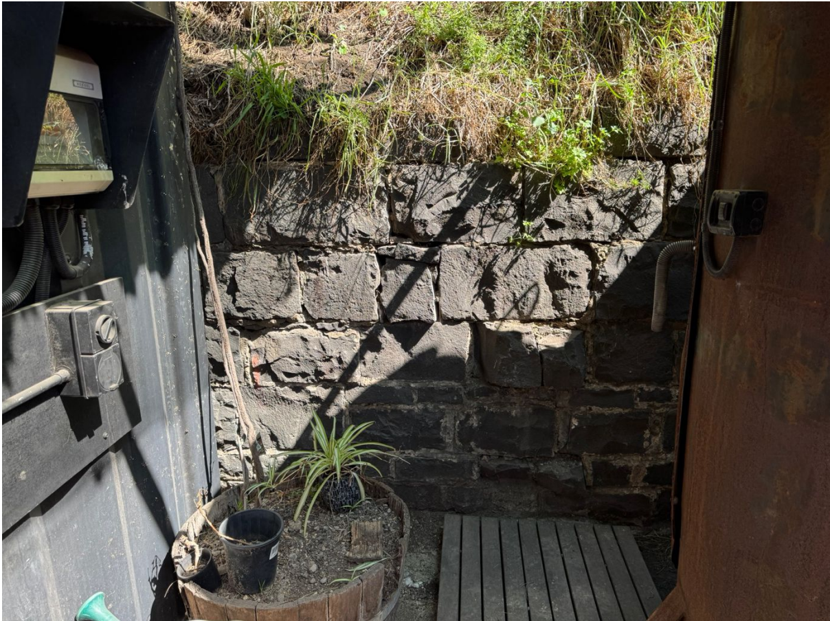
Figure 5: Photograph of the exposed bluestone retaining wall within the Waterside Metal Art site
