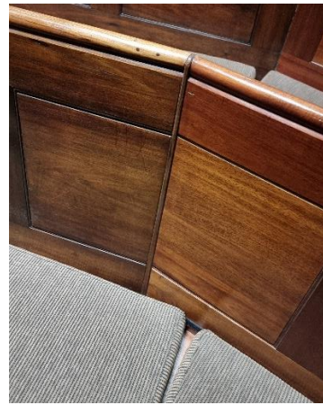
Figure 16 Choir stalls in their current curved arrangement. Note: physical evidence of altered/joined back panels. Source: Trethowan Architecture, 2024.
