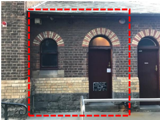
Figure 11 Single-storey addition to north east corner of building as viewed from St. Michael's Walk (east elevation). Part of wall that is primary significant and possibly part of an earlier addition indicated in red. Source: Trethowan Architecture.
