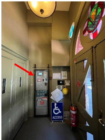
Figure 35 East Lobby looking towards north wall. Note fire indicator system indicated by red arrow. Source: Trethowan Architecture, 2024.
