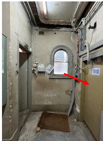
Figure 36 Switch Room looking towards east wall. Note existing opening to East Lobby indicated by red arrow. Source: Trethowan Architecture, 2024.
