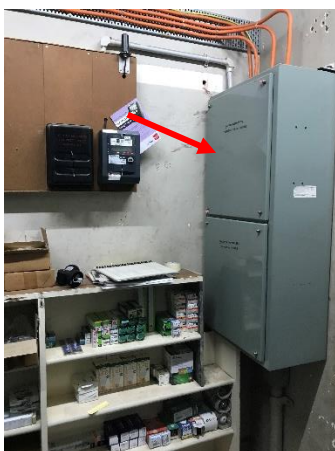
Figure 38 Power supply unit located in north-east corner of the switch room. Source: Trethowan Architecture, 2024.
